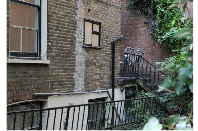
Existing rear elevation showing poor outlook from basement
