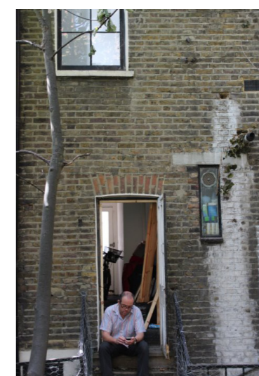
Poor condition of fabric; small window openings
