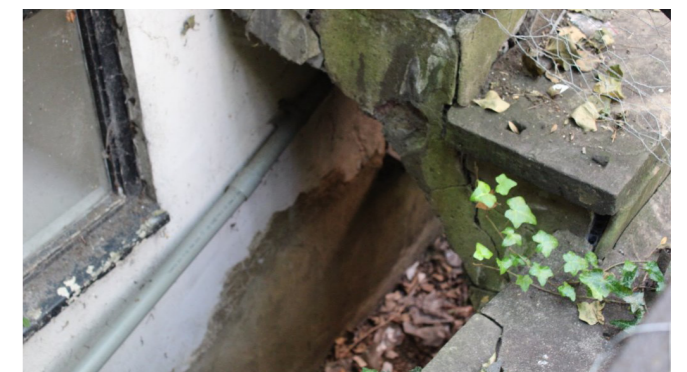
Poor condition of rear steps; no level thresholds
