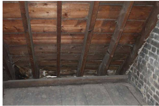
P6 Main roof void showing wooden sarking and daylight at eaves (potential bat access point into void)
