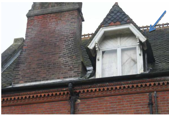
P3 Gap between bargeboards and tiles on northern elevation
