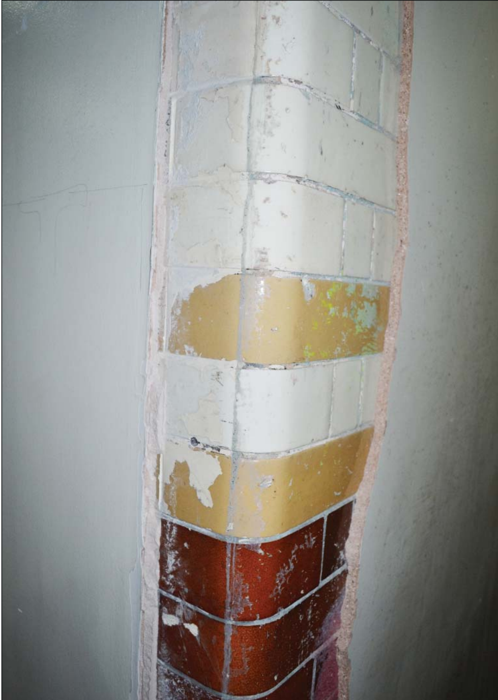
16. Damaged brick faces
