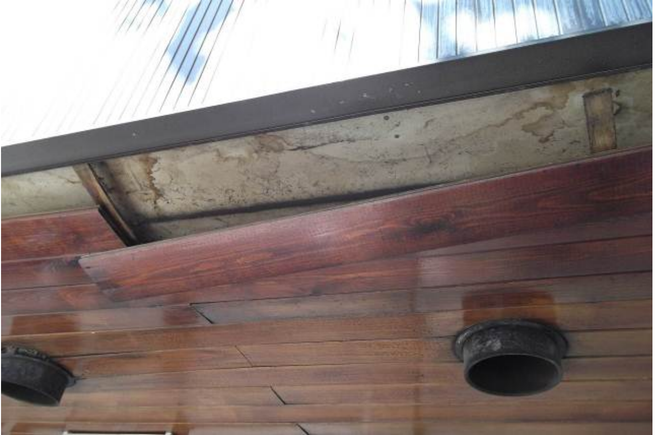
Plate 12. Loose wooden batten beneath porch that leads into entrance of building on Camden Road.
