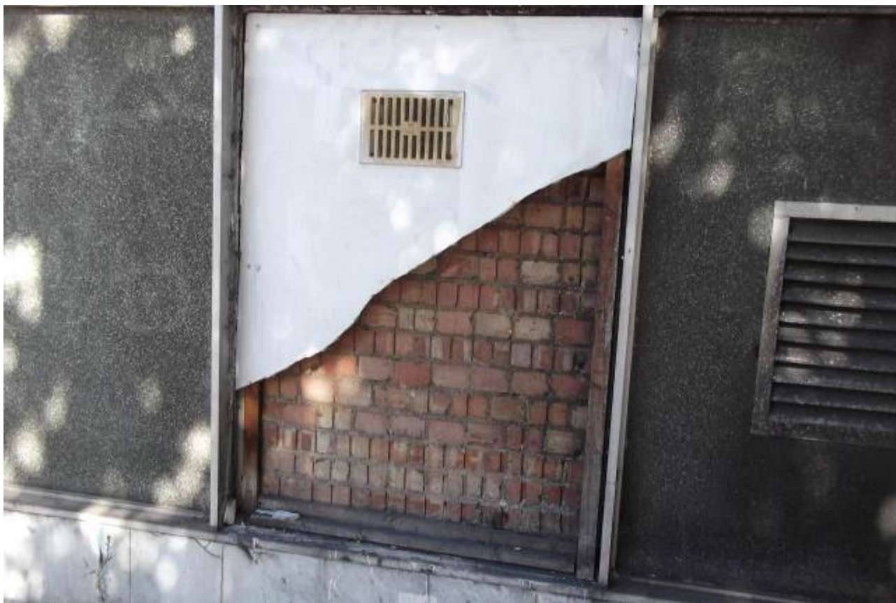
Plate 14. Broken concrete tile on Camden Road side of building.
