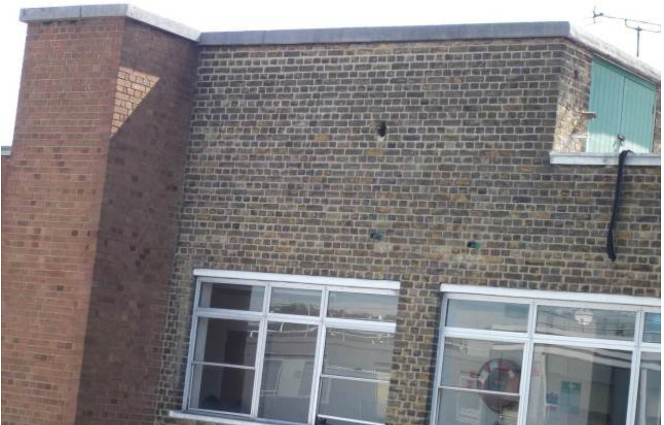
Plate 27. Hole in wall to rear of four storey section of building that overlooks Camden Road.
