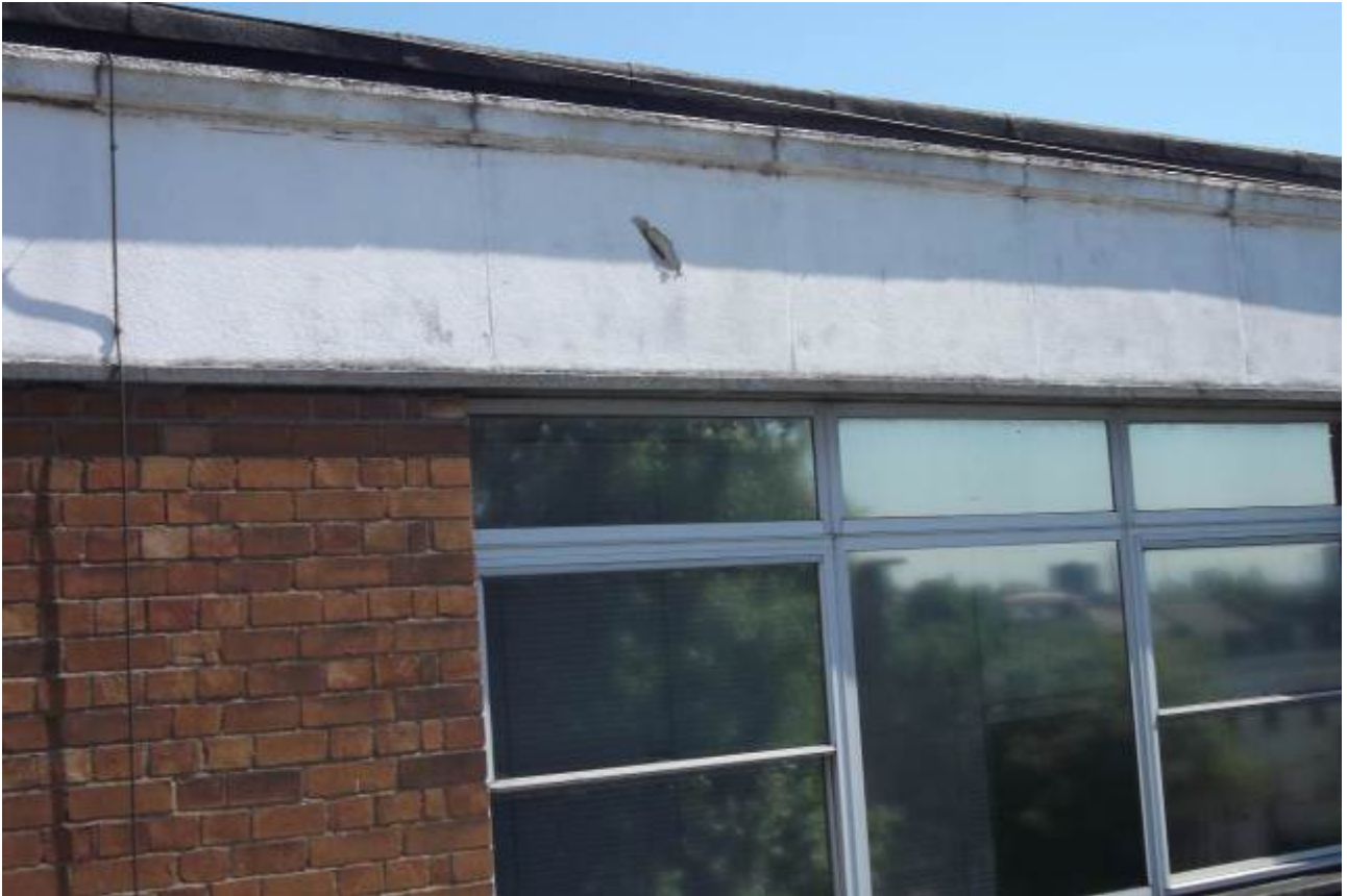
Plate 26. Hole in cement work near roof top.
