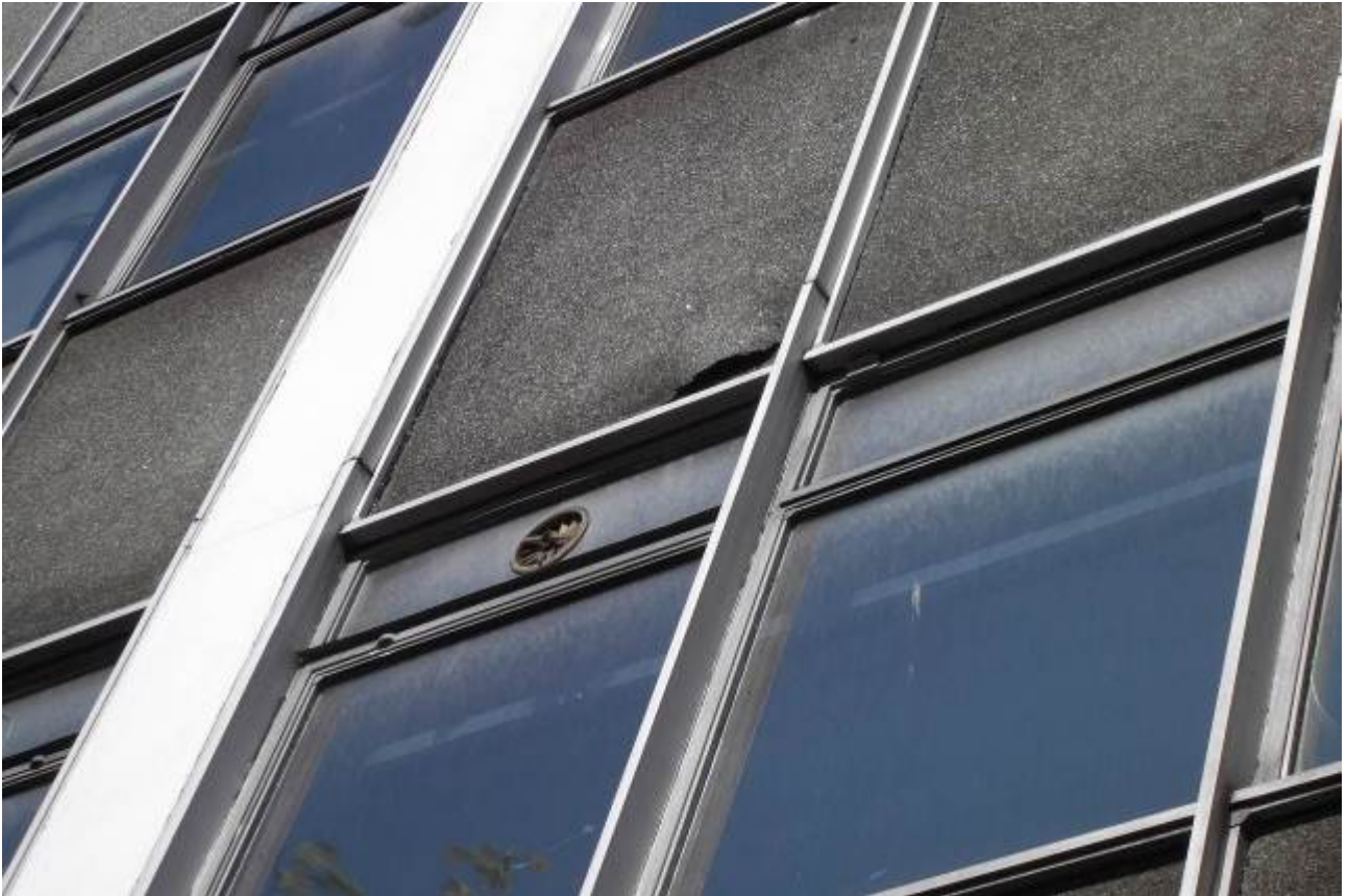
Plate 15. Rip in felt wall tile.
