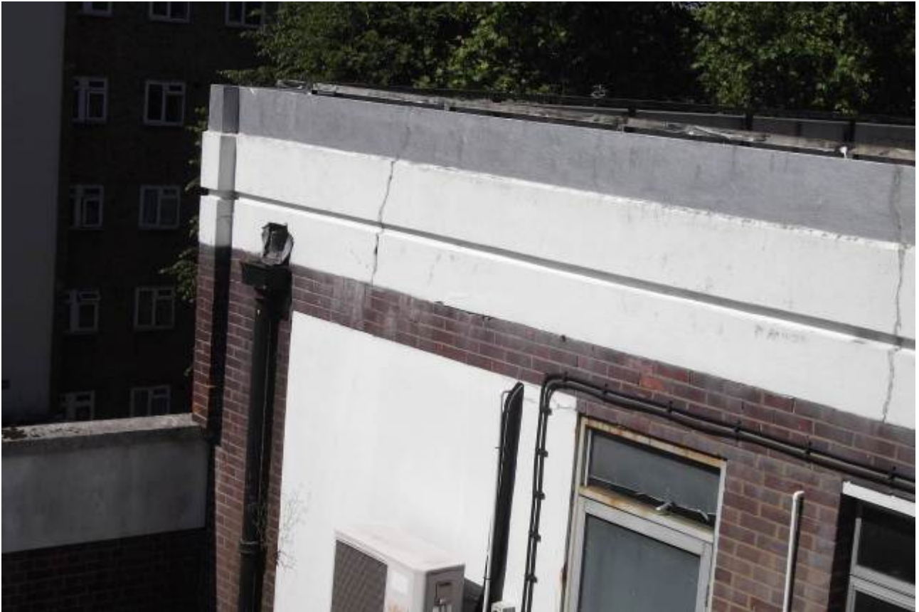
Plate 25. Two cracks in cement work near roof of building.
