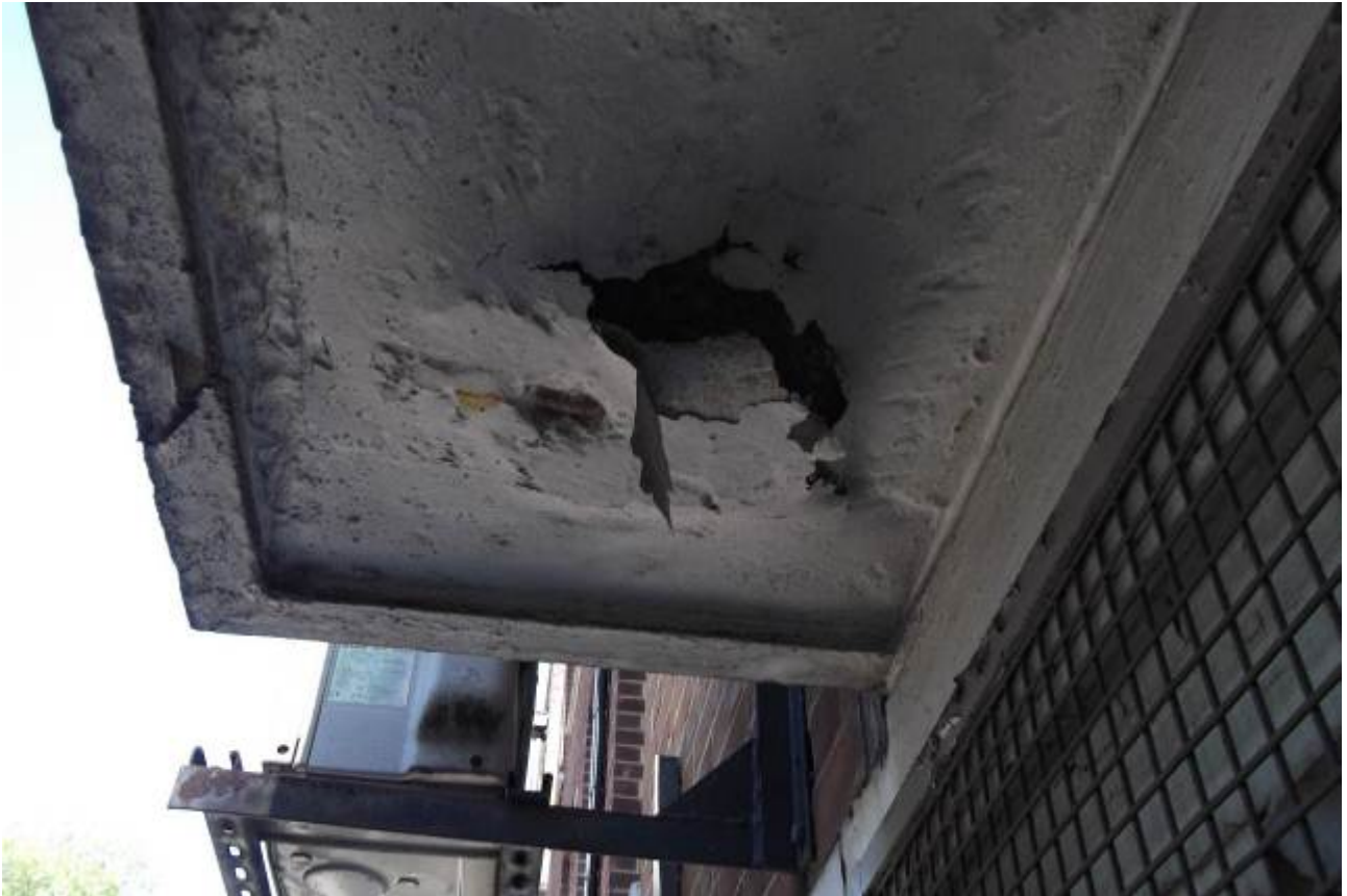
Plate 23. Flaking paint beneath roof of porch leading into basement.
