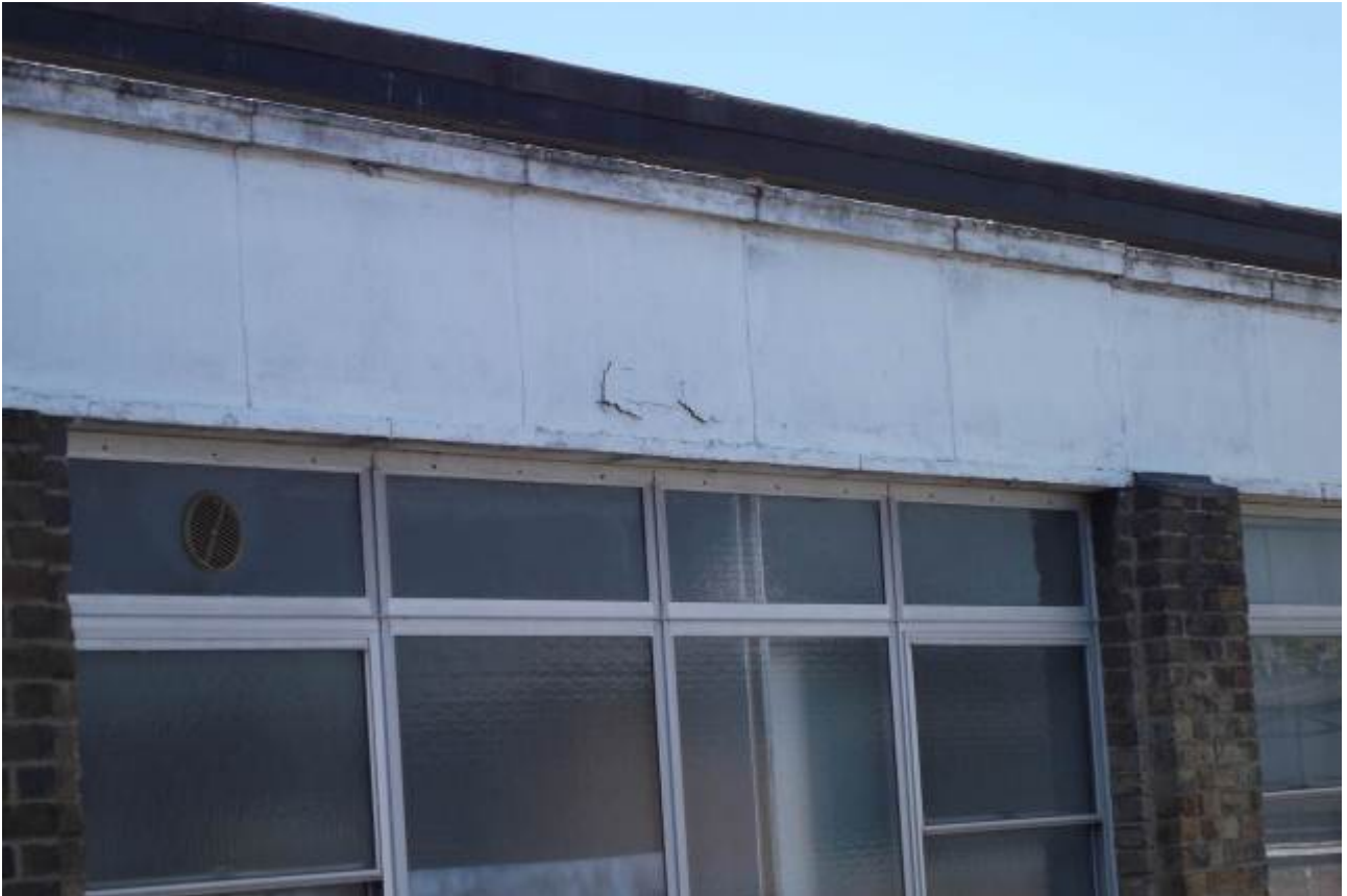
Plate 24. Flaking cement work near roof of building.
