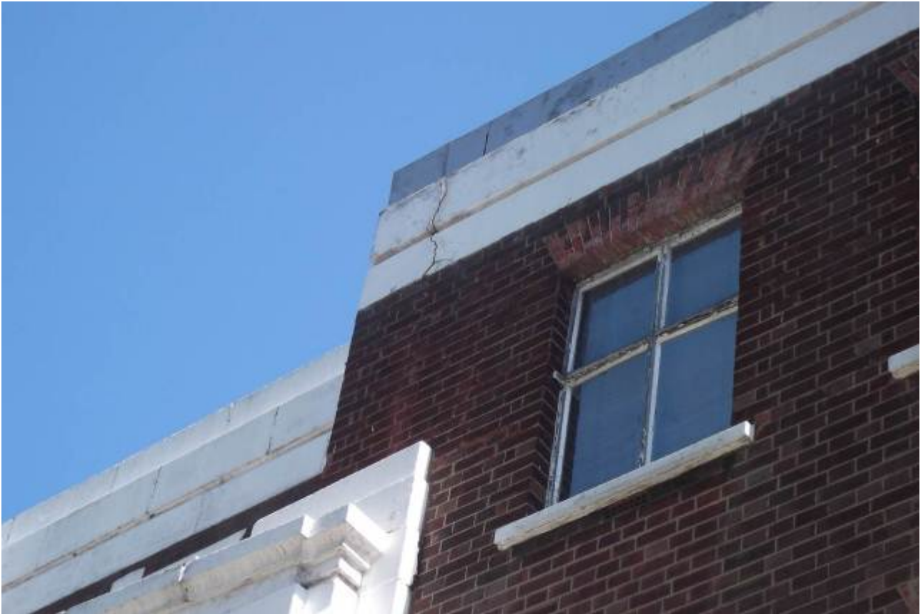
Plate 19. Crack in cement work near top of building located on Pancras' Way side of building.
