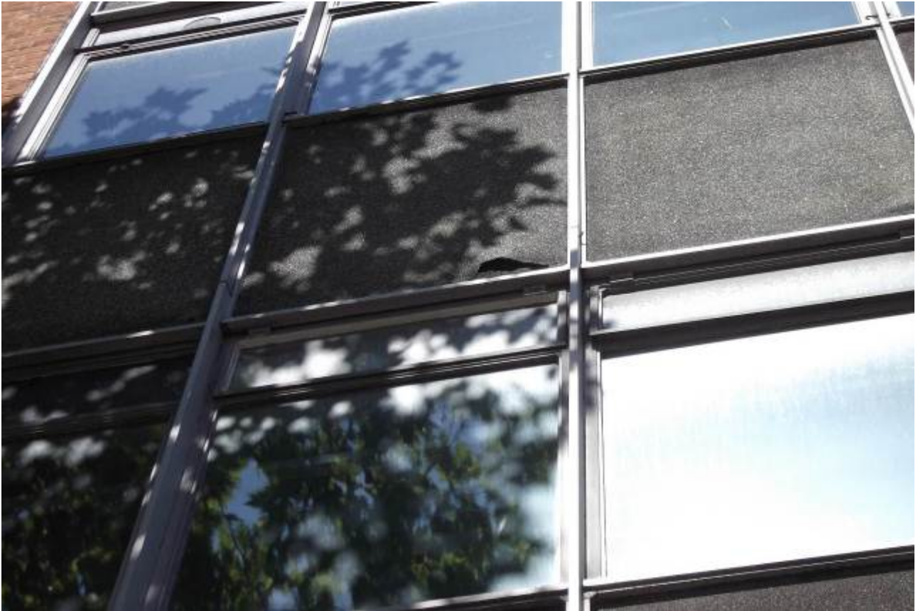
Plate 16. Rip in felt wall tile.
