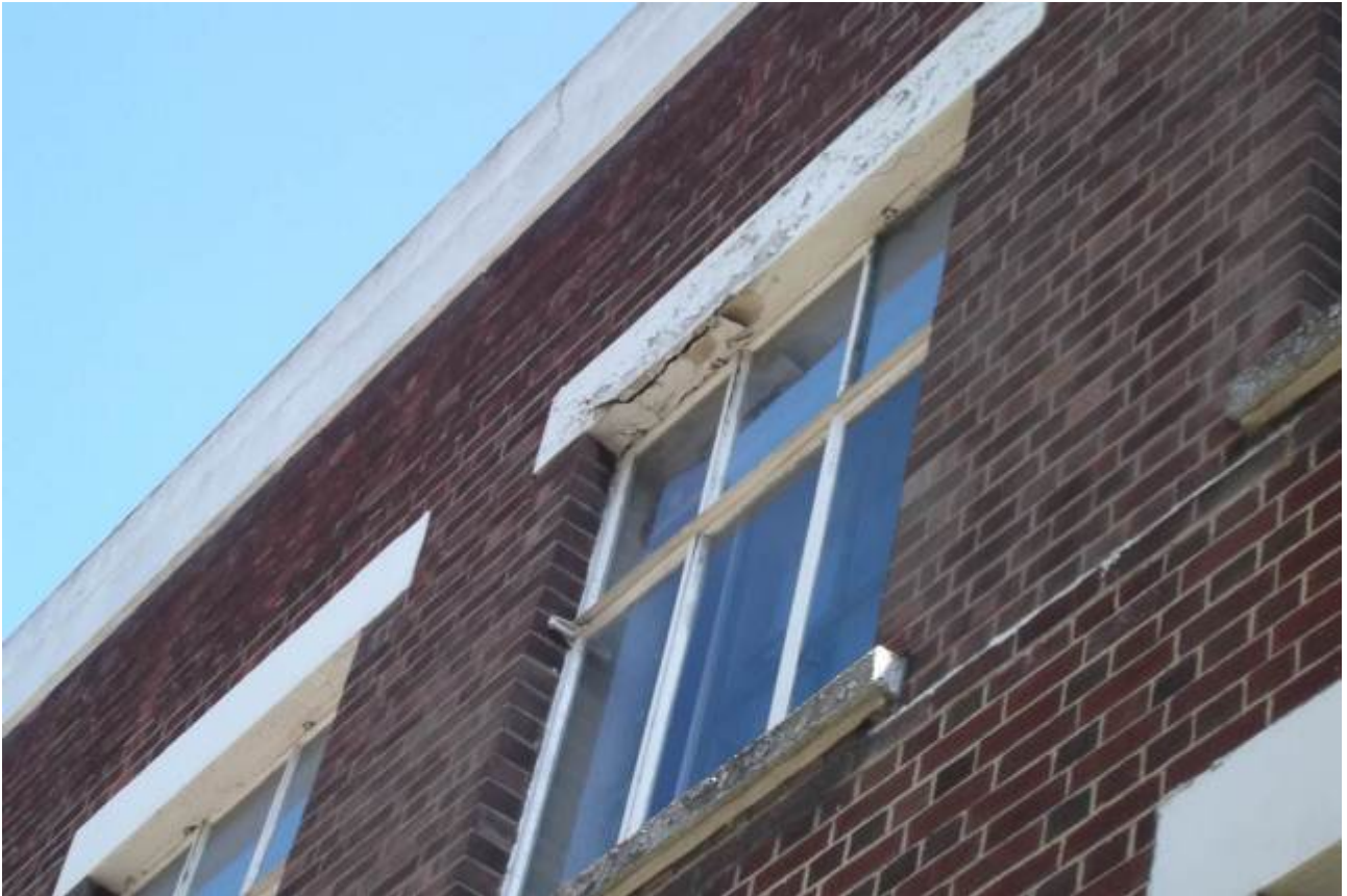
Plate 20. Crack in cement work above window.
