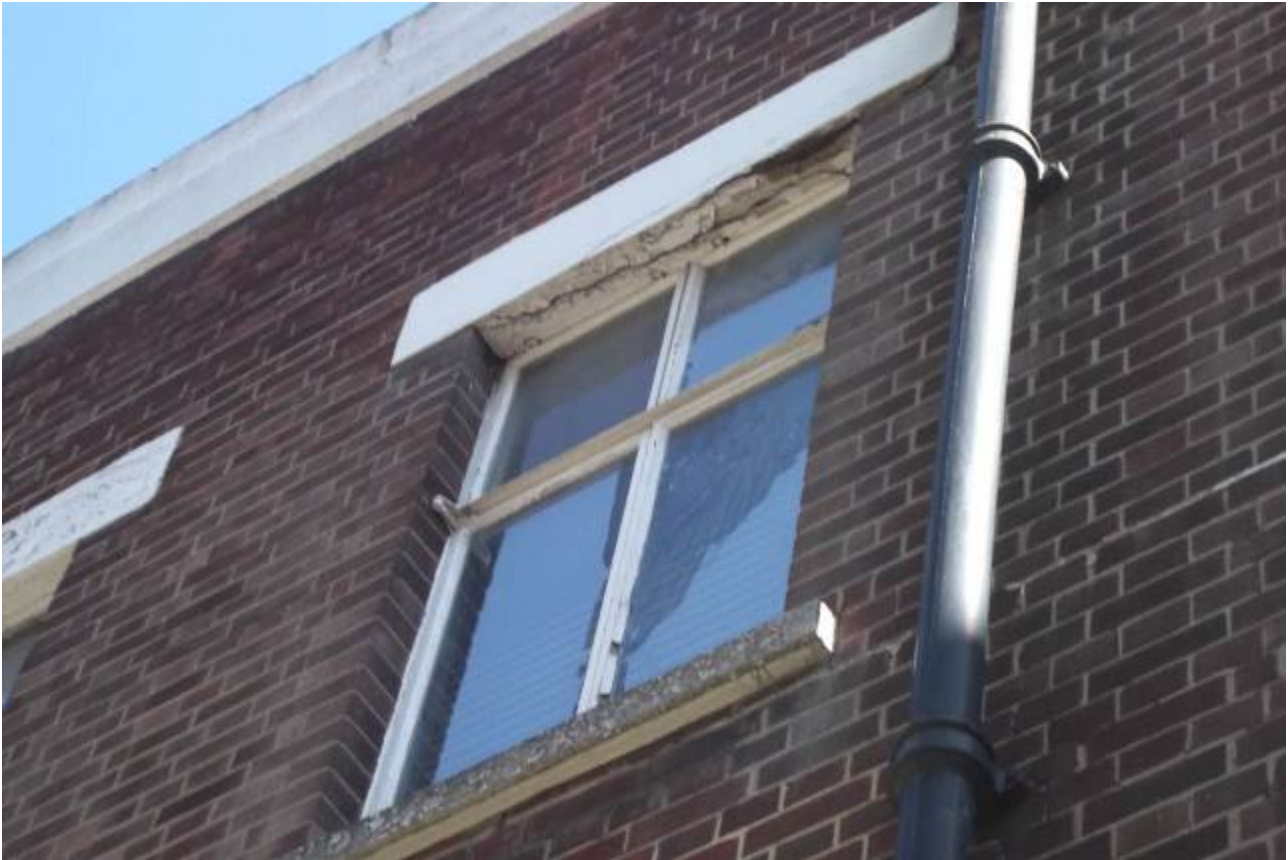
Plate 21. Crack in brickwork above window with large gap.
