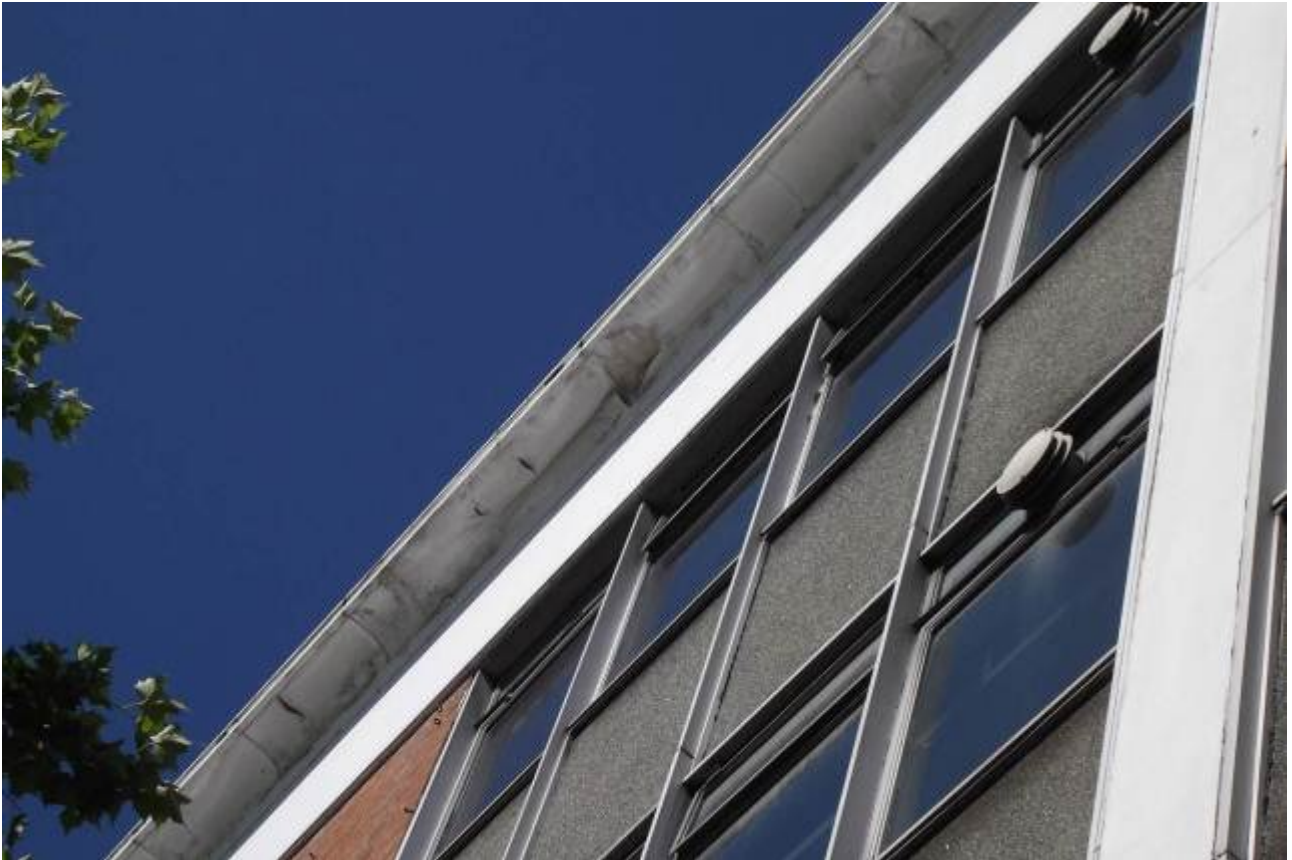
Plate 13. Flaking paint beneath eave of roof on Camden Road side of the building.
