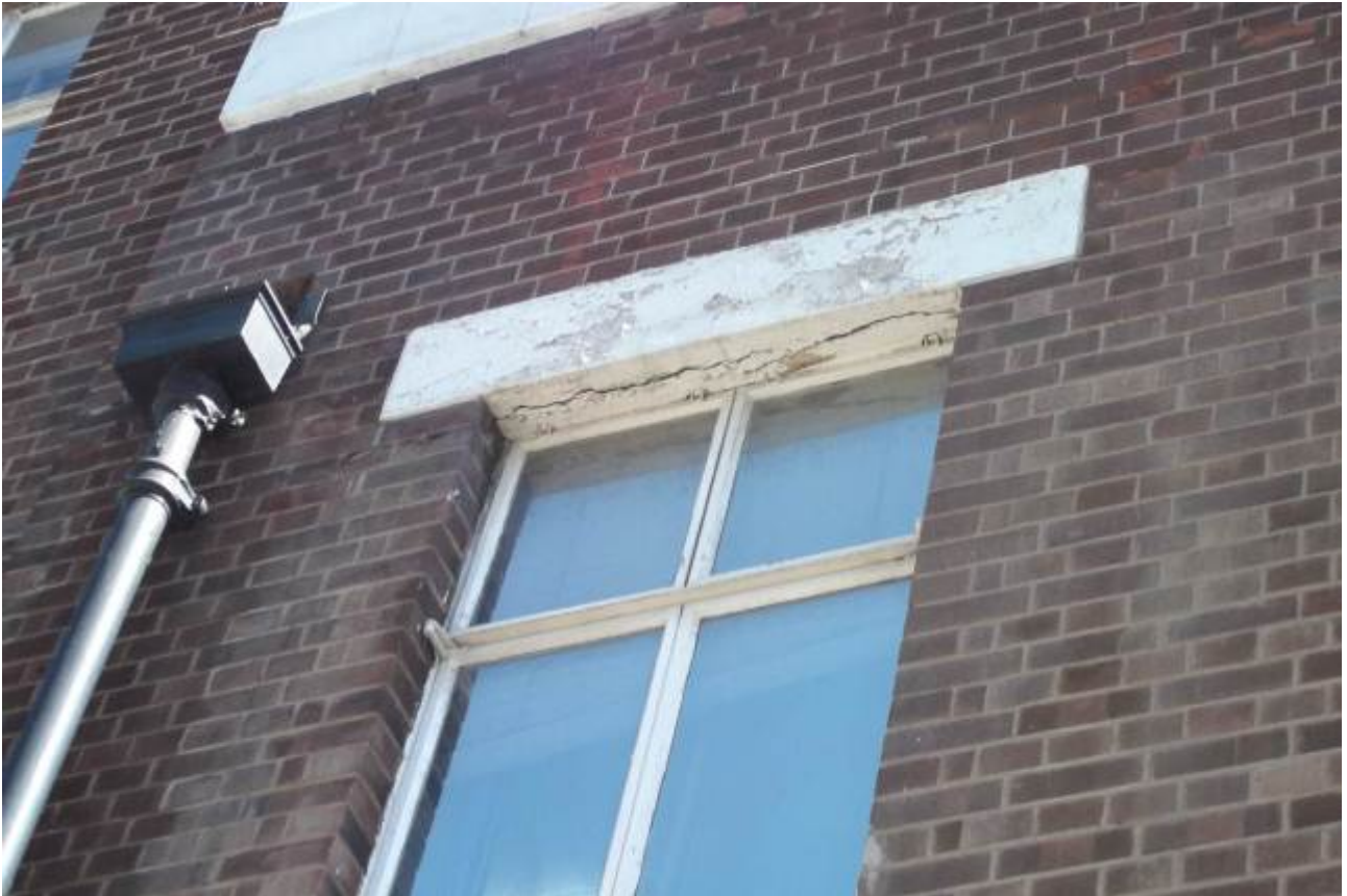
Plate 22. Crack in cement work above window.
