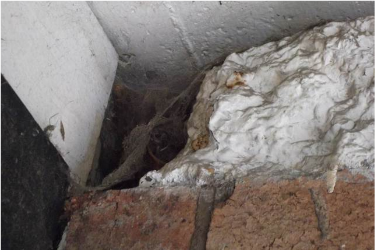
Plate 18. Gap above brickwork in arched entranceway leading onto Rochester Place.
