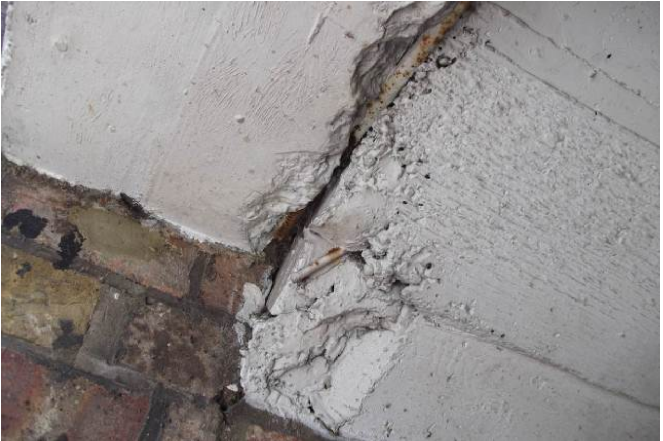
Plate 17. Crack in brickwork above arched porch leading onto Rochester Place.
