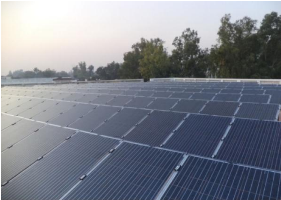
Figure 7 - A typical rooftop photovoltaic array
