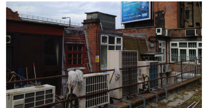
Figure 26: A photograph of the condition at the rear of the properties at 11-12 New College Parade. The additions that have accrued over the years detract from the architectural integrity of these buildings.
