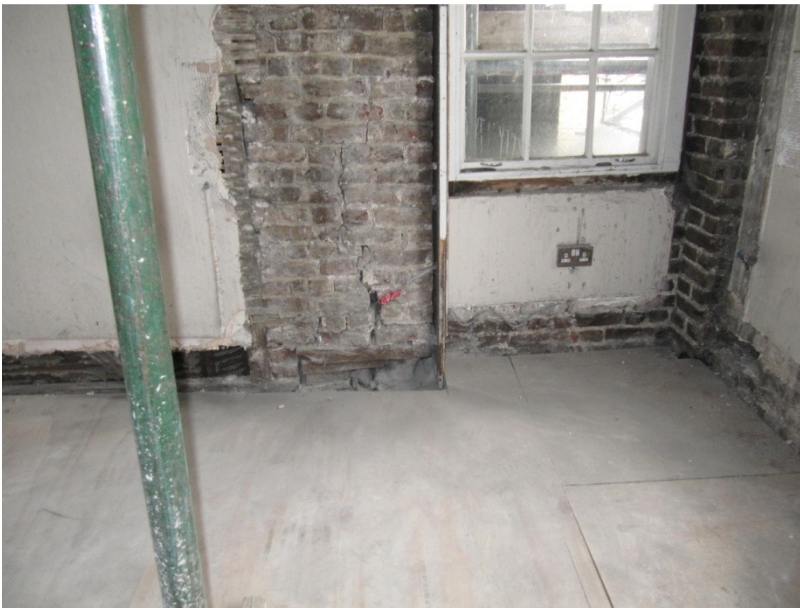
Photograph 3. Cracking in rear wall adjacent to stair case.
