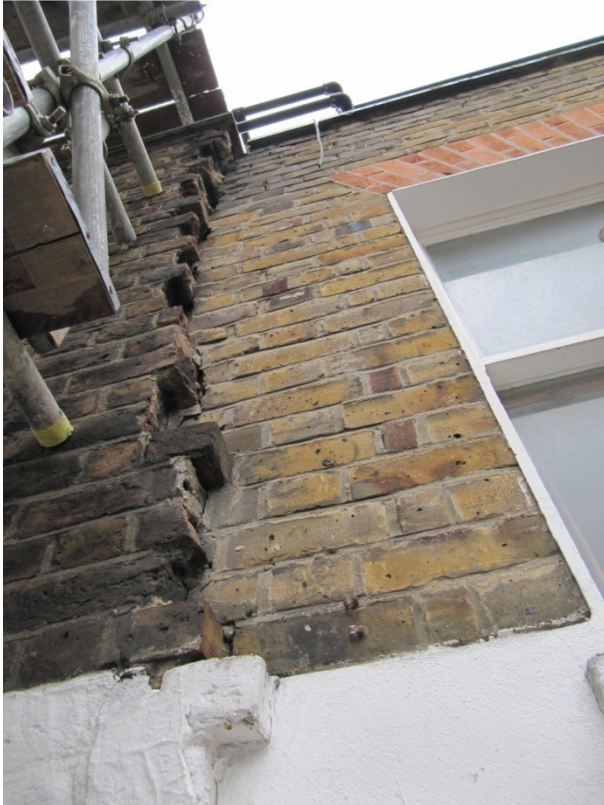
Photograph 2. Dislocation of front elevation from Party wall.
