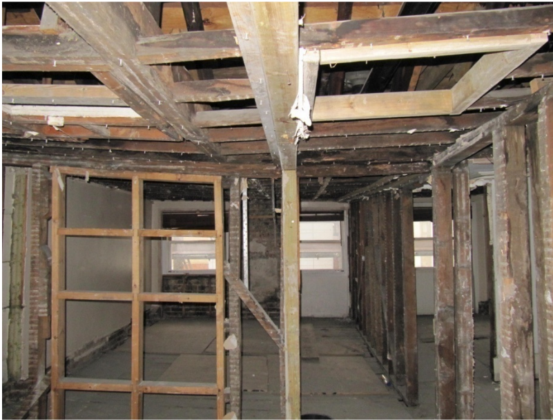
Photograph 1. Third floor showing deformation in the roof timbers.
