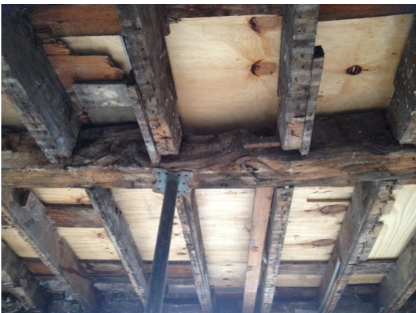
Existing joists poorly connected to existing beam
