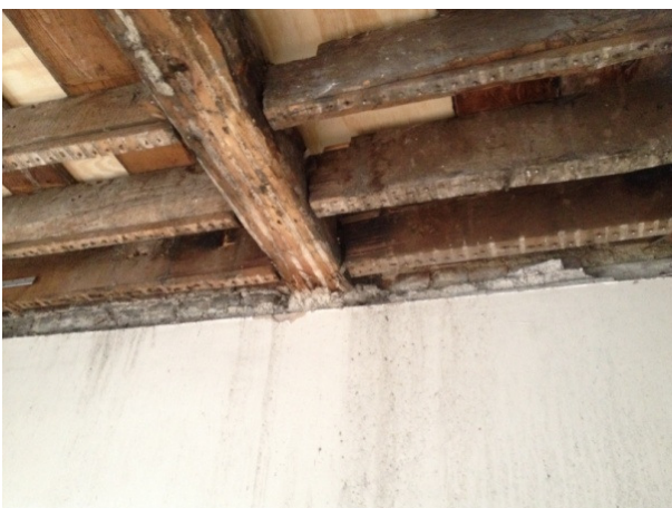
Existing joists over-notched
