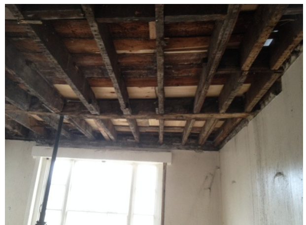
View to underside of 3 rd floor showing excessive floor deflection
