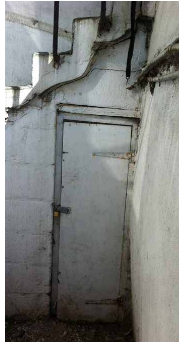
Fig 1.2.9 Condition of stairs and external walls
