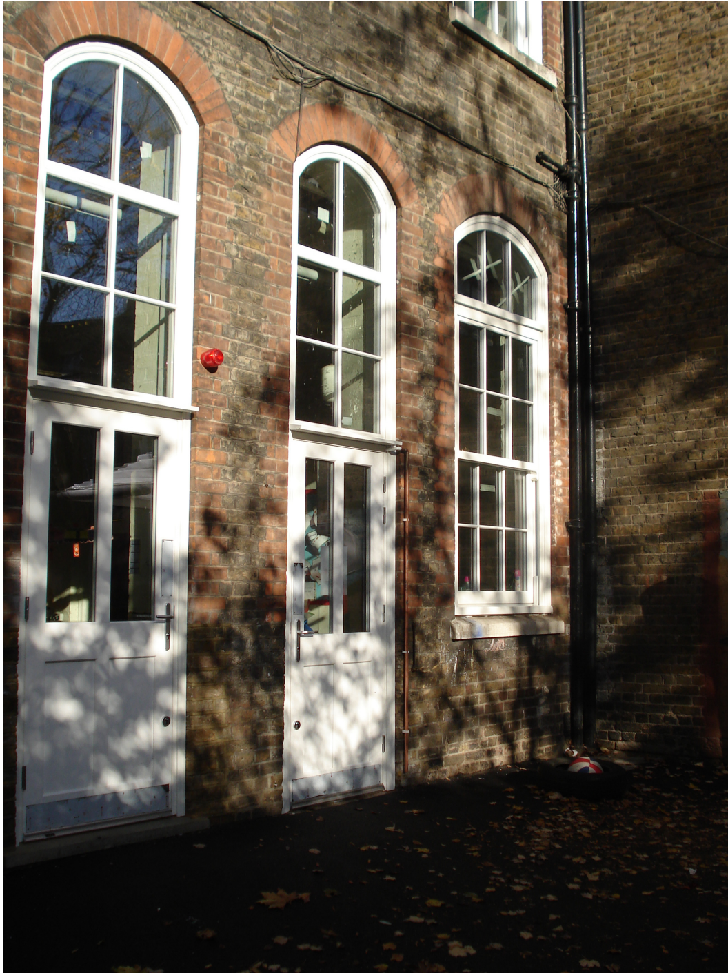
Windows on western side of the elevation where canopy is yet to be installed.
