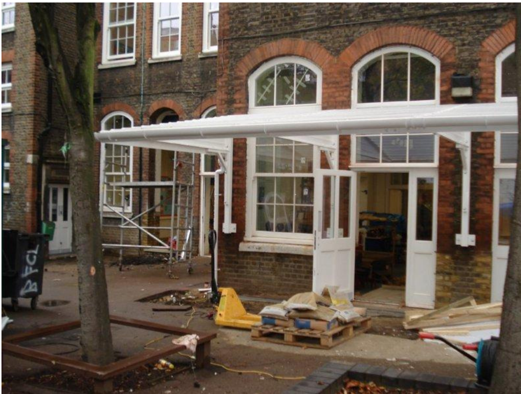
Canopy as installed on the eastern side of the elevation.
