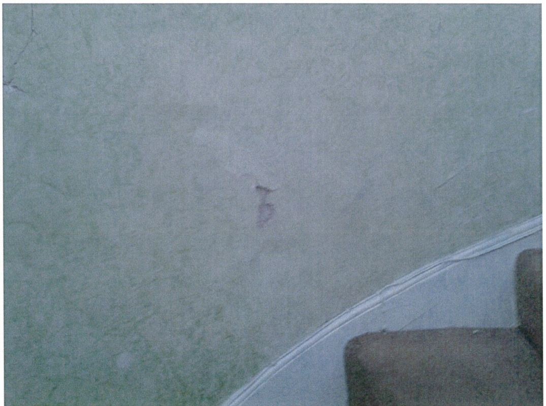
Photograph 7 – Further cracks in stairwell
