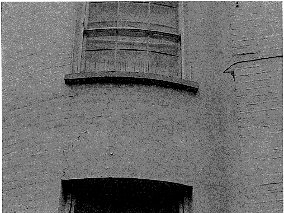
Photograph 5 – Cracks in painted brick over windows at first floor
