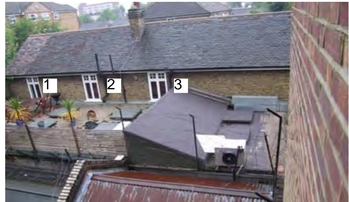
Crowndale House Windows
