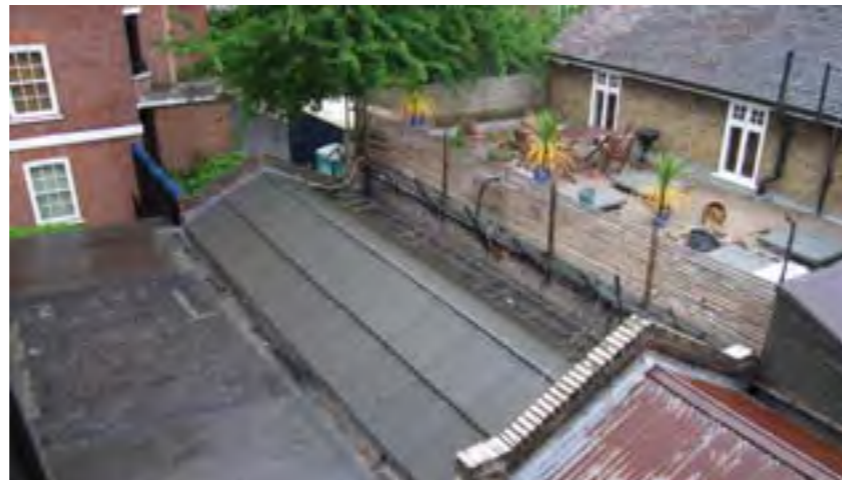
Roof of existing garages to be demolished (flat portion) and property behind
