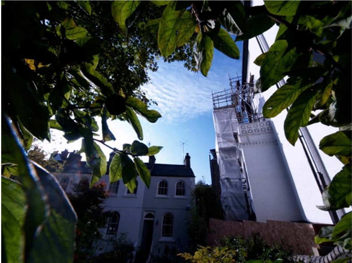
Figure 16 - Dr Swain's photograph PA160049 taken on 16 October 2008 showing work underway on the Rear Extension (under the scaffolding), but not yet commenced on the Staircase Extension. The northern lean-to is still standing.
