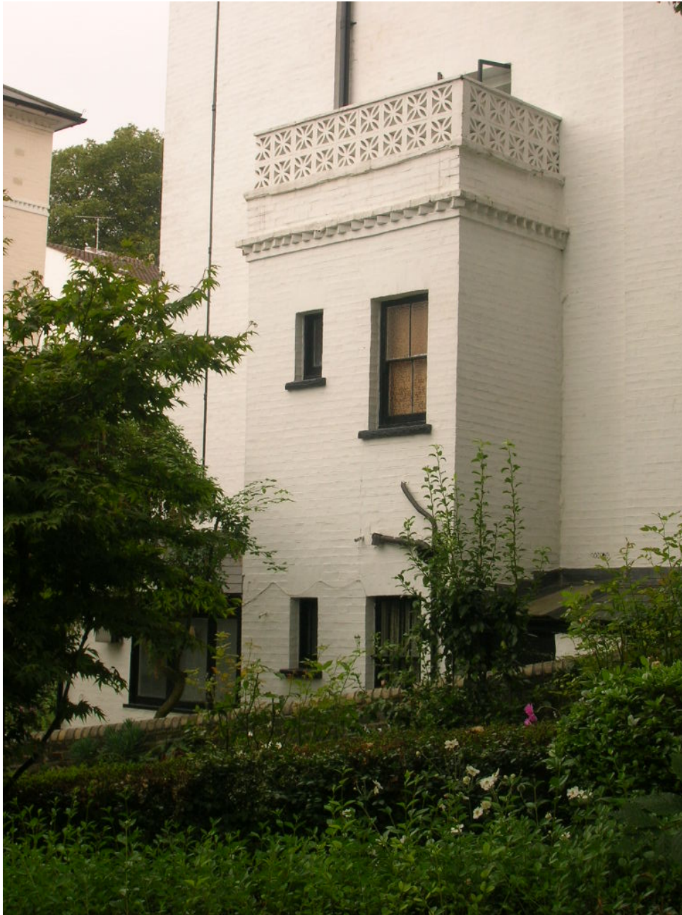
Figure 7 - Photograph taken by Council officer on 8 August 2008. The northern lean-to is visible on the right and the window of the southern lean-to on the left.
