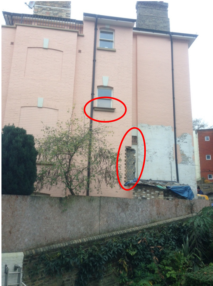
Figure 26 - View of the rear of the property taken on 5 December 2013 showing that the Stairway Extension is still not complete. Note that a protective board remains on top of the (composite) stone window sill. A large chunk of the wall remains missing, to accommodate the (rejected) second storey to the WC Extension.
