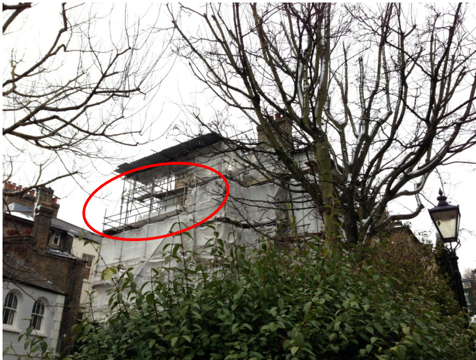
Figure 25 - Photograph of the rear of the property taken on 25 March 2013 - note that the balcony above the Rear Extension is not complete as the railings have not been inserted - the rest of the rear remains tightly covered in tarpaulins.
