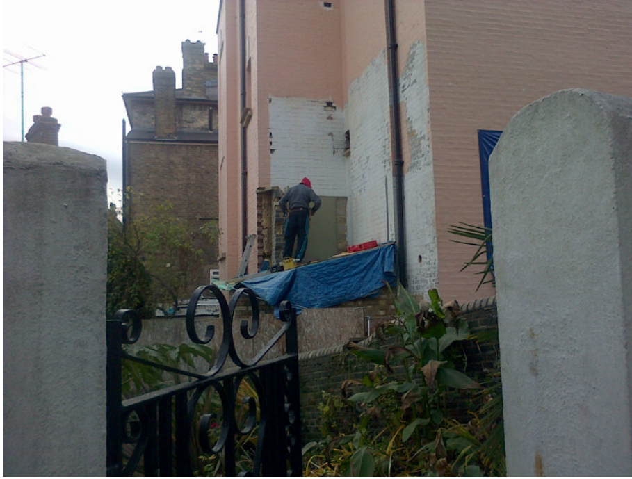
Figure 27 - View from Willow Road taken 4 December 2013, again showing the incomplete Staircase Extension.
