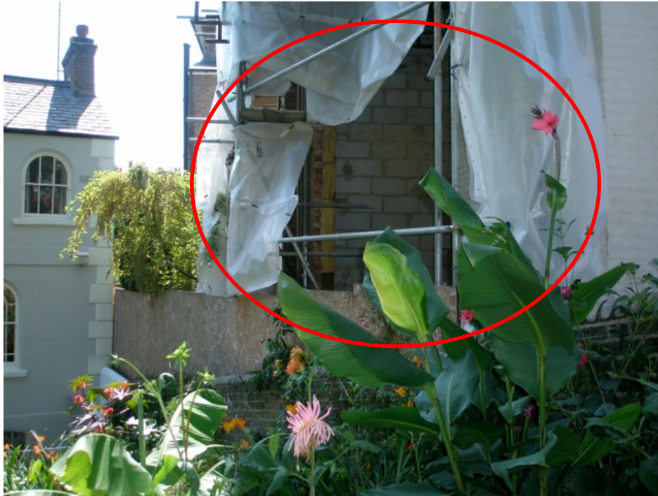
Figure 24 - Dr Swain's photograph P8165779 of the rear of the property taken on 16 August 2010 showing the breeze block construction of the Staircase Extension.
