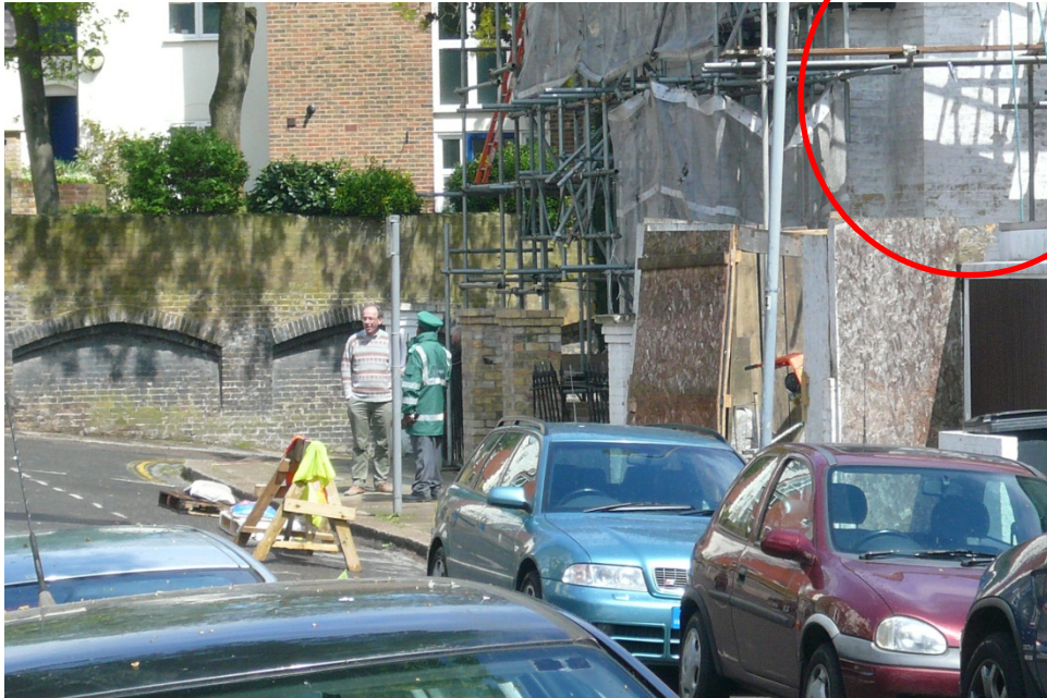
Figure 31 - Photograph taken on 9 May 2013 showing the dilapidation to the tarpaulins at the front of the building. Mr Galway-Cooper is shown talking to a parking officer. Note also the unapproved blocked off parking bays.
