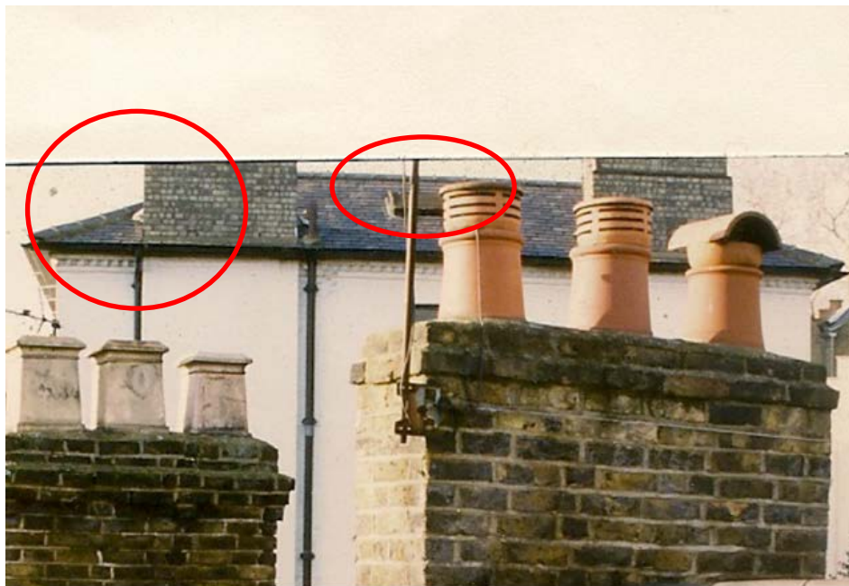
Figure 11 - Photograph of the rear roof of the property taken before the works began. There is no satellite dish or antenna shown on the left hand chimney in the background. Note also that the skylight has now been removed.
