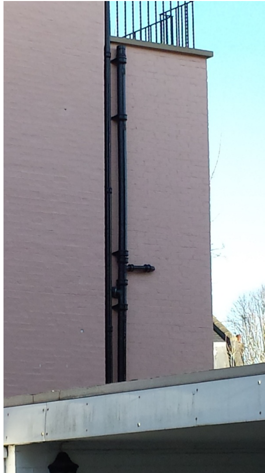
Figure 23 - Photograph taken on 29 December 2013 from Gayton Crescent showing the side of the Rear Extension. The soil/vent pipe (on the right) is new (as are the bricks to which it is attached). Note also the balcony railing. Note that the soil pipe vents directly under a balcony outside double doors i.e., effectively into a bedroom of the property.
