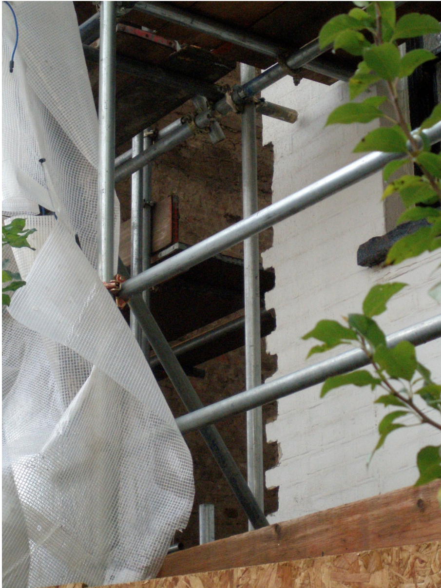
Figure 19 - Dr Swain's photograph P1012268 taken between 28 October and 11 November 2008 showing the then existing central protrusion at ground floor level. The jagged brick work is to accommodate the Rear Extension connecting to the central protrusion (Staircase Extension).
