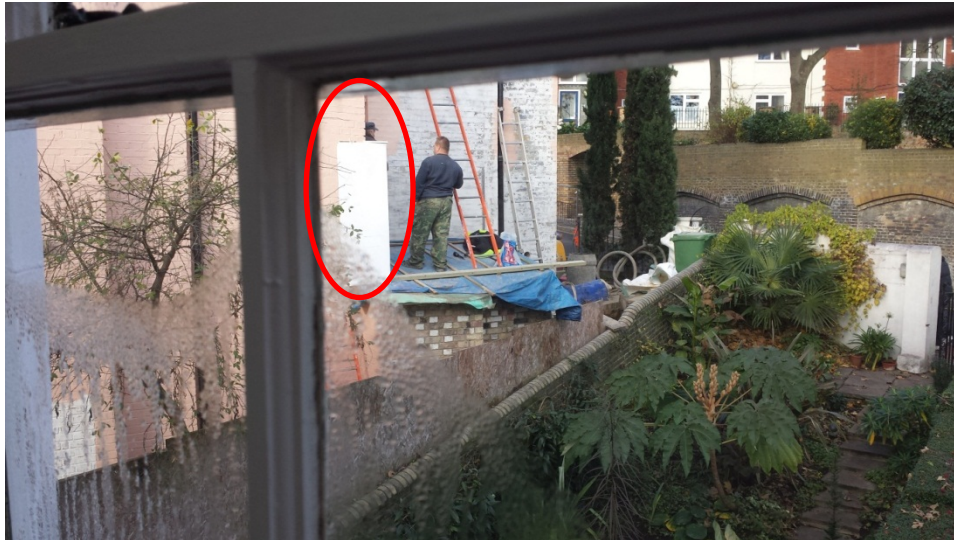
Figure 29 - View of the rear of the property taken in December 2013, showing men working above the roof of the WC Extension. The missing part of Staircase Extension has been covered with white plasterboard.
