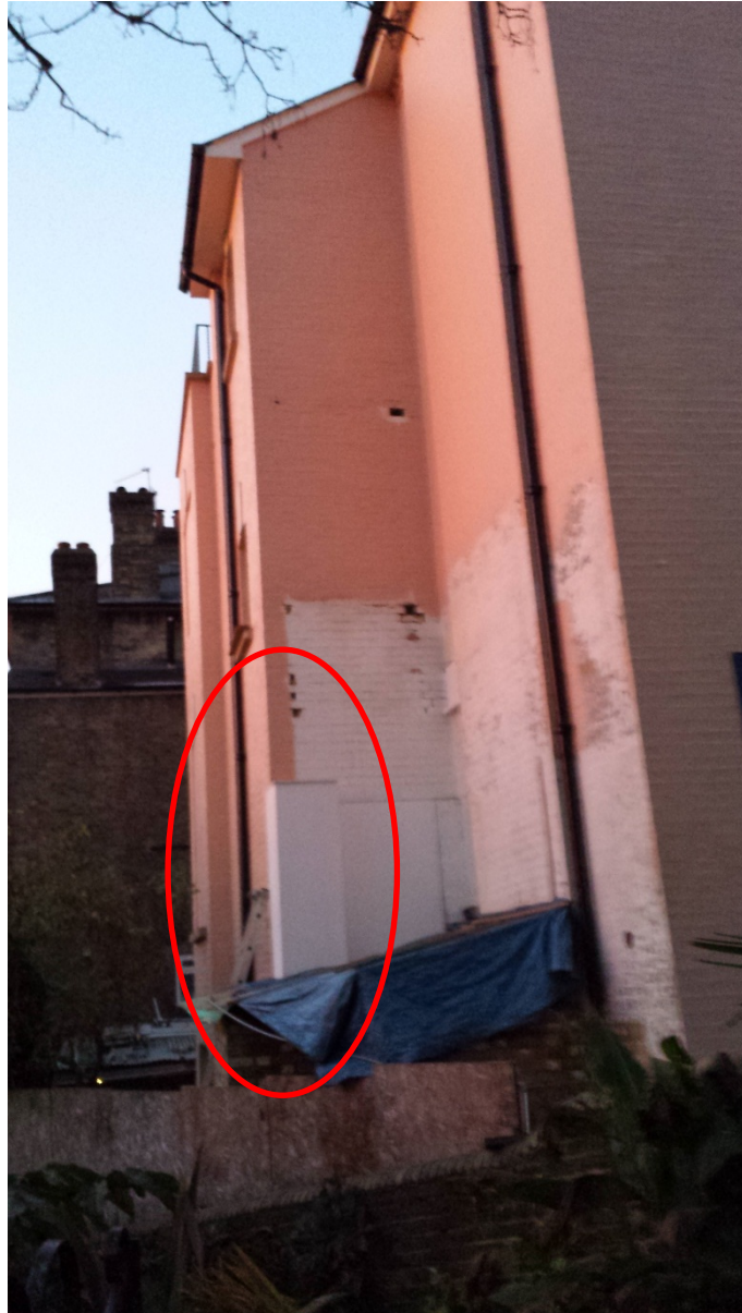
Figure 28 - View of the rear of the property from Willow Road taken on 5 December 2013, showing the incomplete Staircase Extension, with bricks missing. One gap in the bricks has been covered by white plasterboard, later to be painted trout mousse.
