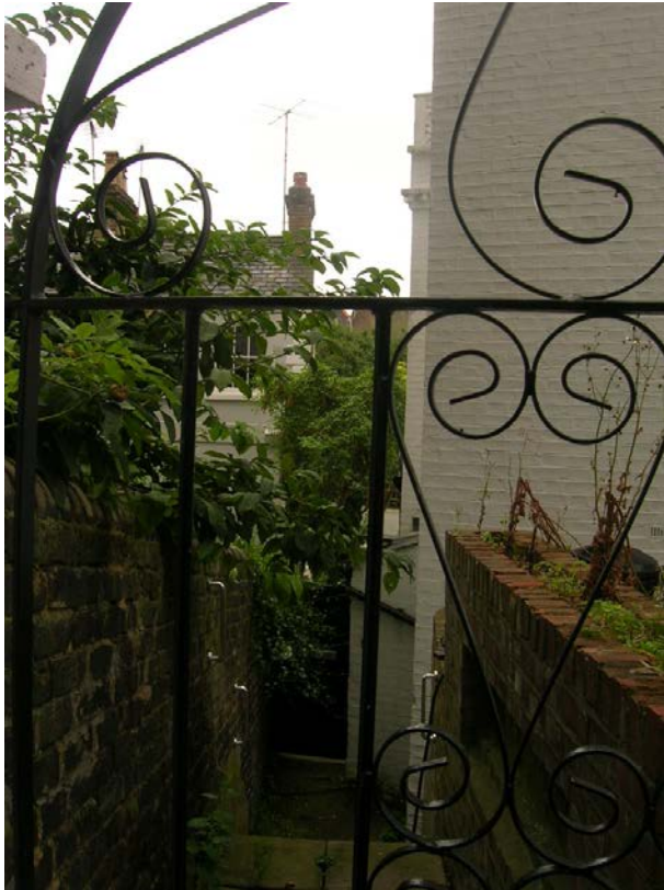
Figure 9 - Photograph taken by Council officer on 8 August 2008 from Willow Road, looking along the 15 Gayton Crescent side of the boundary wall with 41 Willow Road. Note in particular the gap between the wall and the building, which has since been built out. 41 Willow Road is visible.
