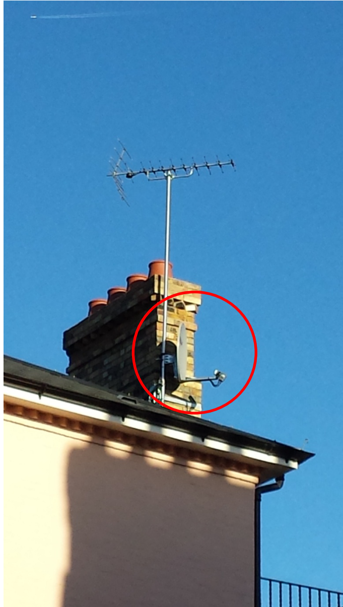
Figure 12 - Photograph taken on 29 December 2013 from Gayton Crescent showing satellite antenna and dish for which no approval has been sought or given. The railing of the new balcony on the second floor is also shown.
