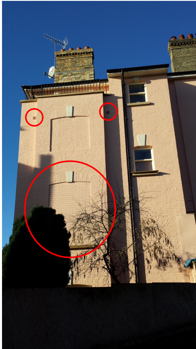
Figure 10 - Photograph taken of the rear of the property on 29 December 2013. Note the lower blind window is made of plaster or concrete with the brick lines hand-drawn. Note also the two extractor fans either side of the upper blind window.
