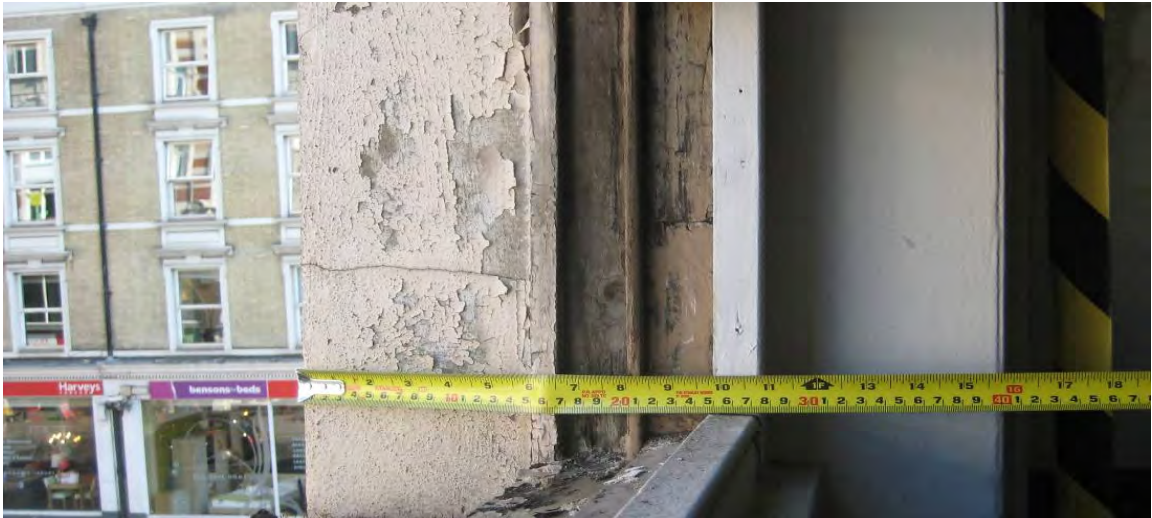
PHOTO 11 - Close up of a typical window sub sill and timber sill. Both sub sill and sill were in poor condition and in need of replacement.
