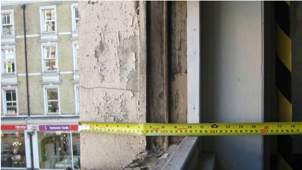
PHOTO 8 - Close up of window reveal and sub sill. Wall thickness varied but window reveal's depth remained constant at approximately 150mm. Paint cracking and peeling.
