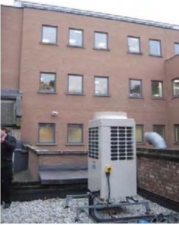
Existing condenser unit
