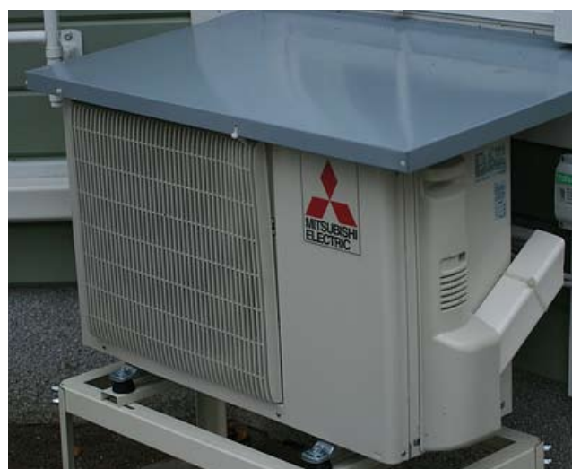
ASHP external unit
