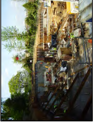
SAMPLE PICTURE OF BASEMENT WORKS DESIGNED BY TAYLOR WILLET SPINRAI VEITCH ROAD, HAMPSTEAD, NW3
