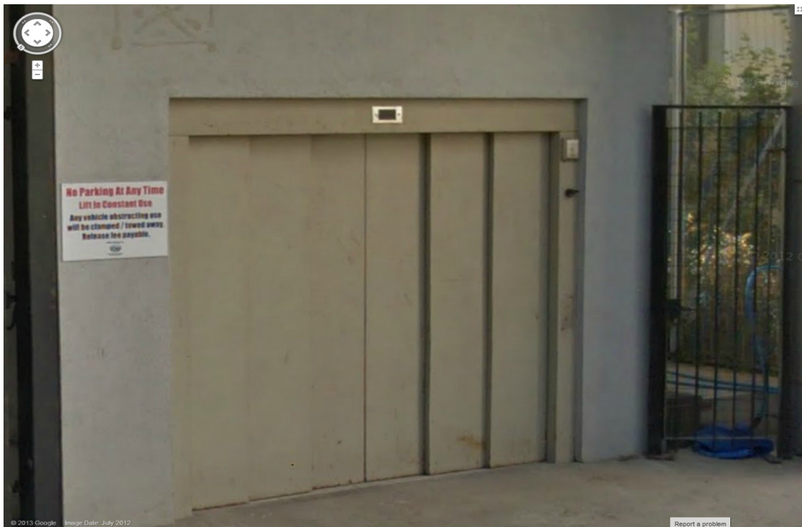
Fig 2 – Photograph showing an example of car lift entrance doors finished in RAL 7038.
