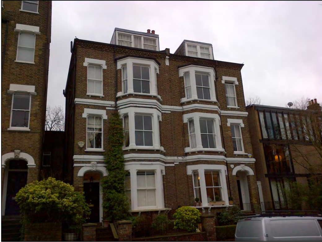
Photograph One: Front view of 35 and 33 South Hill Park. Note the strapping above and below bay windows of No. 35. No. 33 has had them mostly removed, but wall bolts still remain visible.
