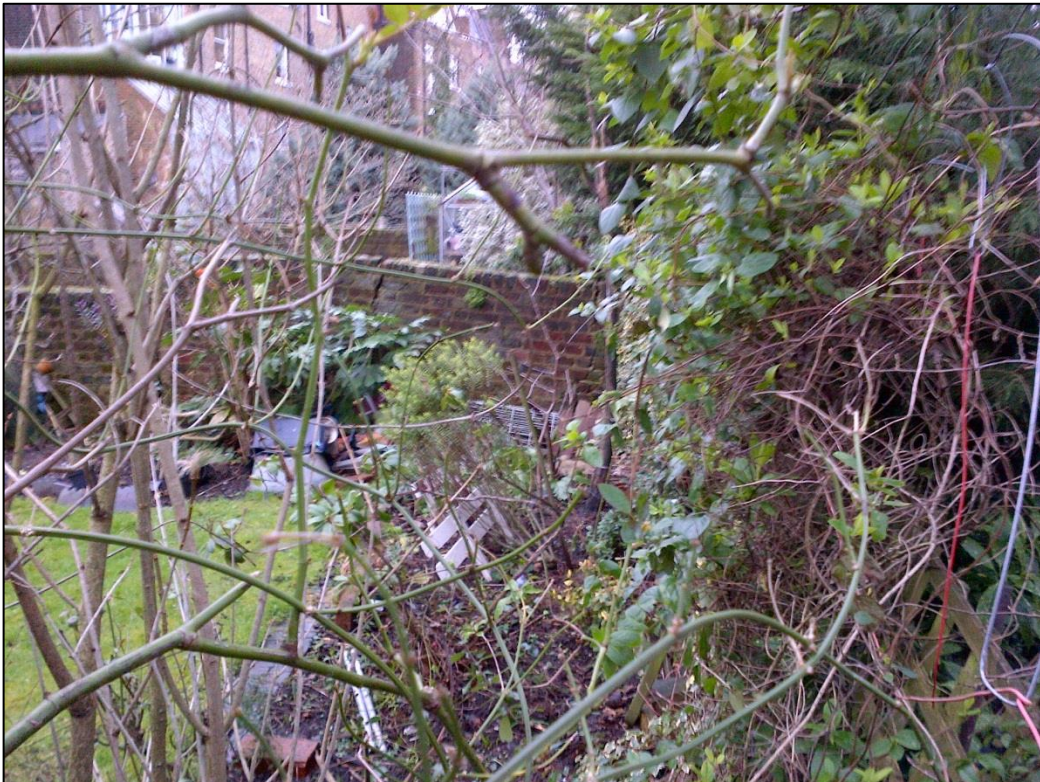
Photograph Two: Garden wall of number 37 South Hill Park showing large crack and leaning towards Parliament Hill gardens
