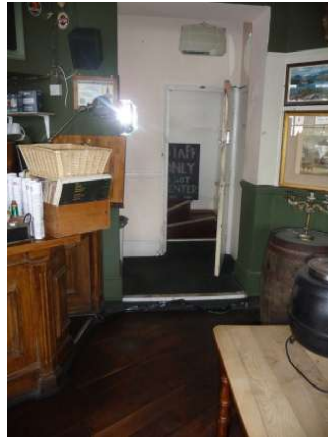
Internal view of existing staircase to upper floors, to be enclosed with new corridor wall.
