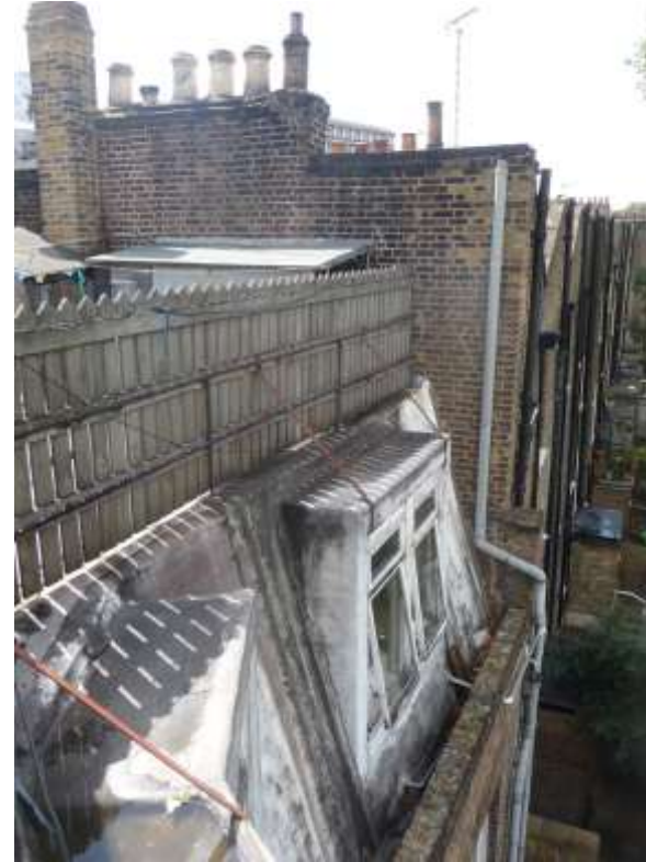
View from roof looking south showing rear elevations of houses on Calthorpe Street
