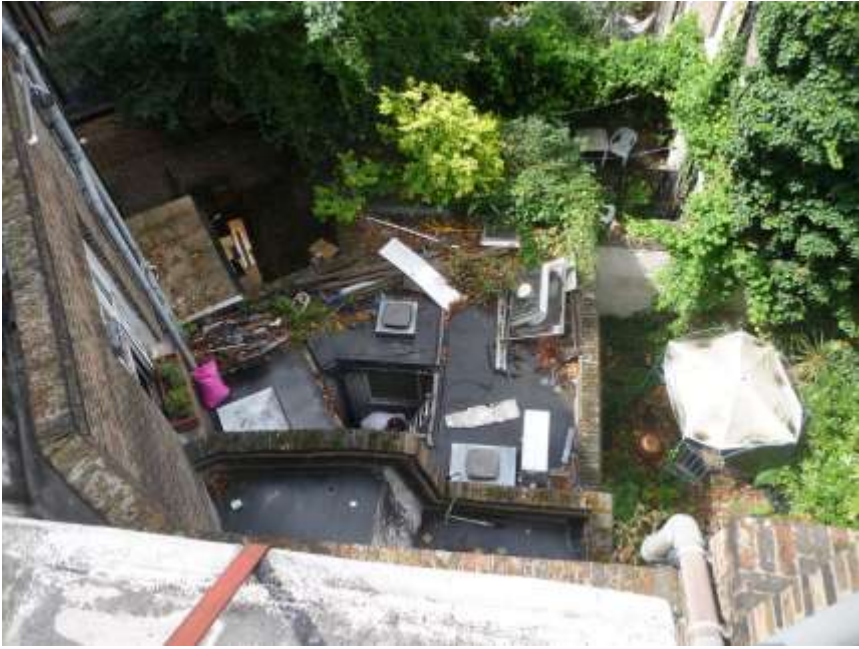
View from roof to Ground Floor rear extension to be demolished and rebuilt.
