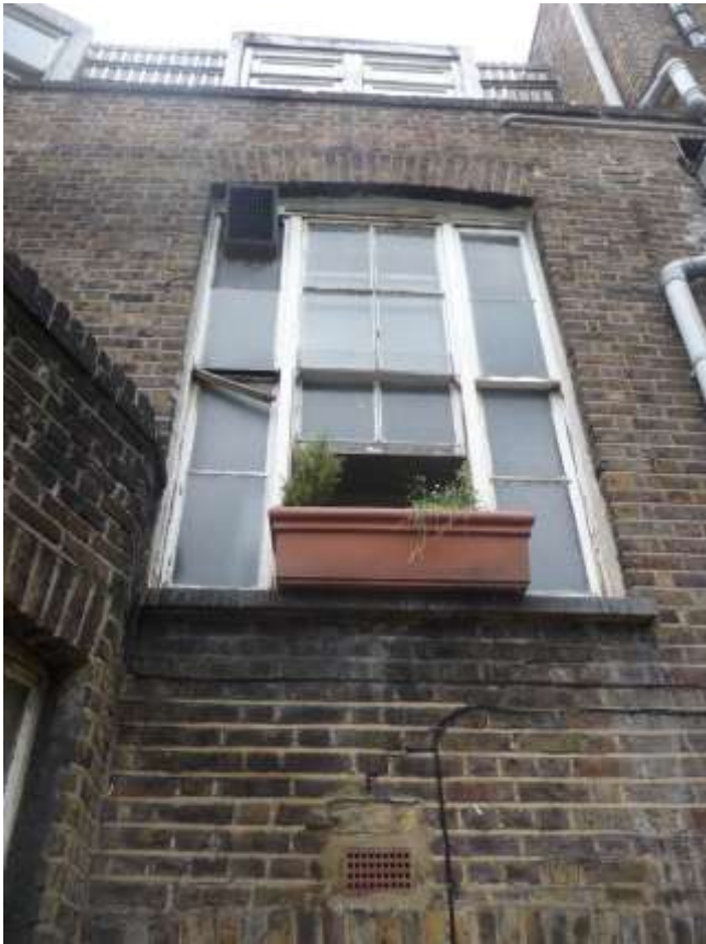
Original window to rear elevation, First Floor and in poor condition.
