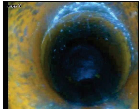
FWMH5X_8aaea2d5-d64c-4bc7-8aee-dac7876d4129_20241007_013734_189.jpg, 00:00:36, 6.00 m Roots, fine at joint
