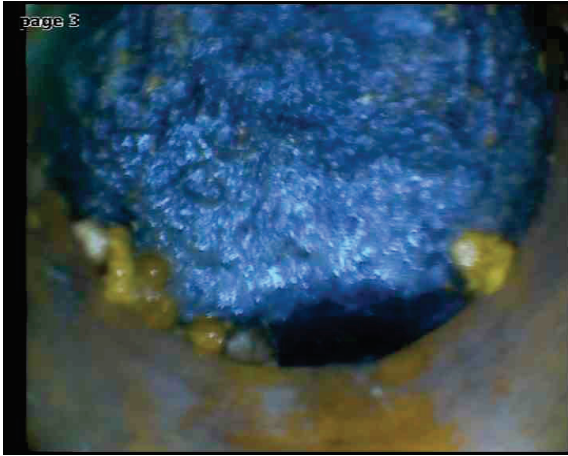
FWMH5X_da81ad58-43de-48ab-ac0c-af8977441448_20241007_013825_178.jpg, 00:00:53, 7.90 m Roots, mass, 90% cross-sectional area loss
