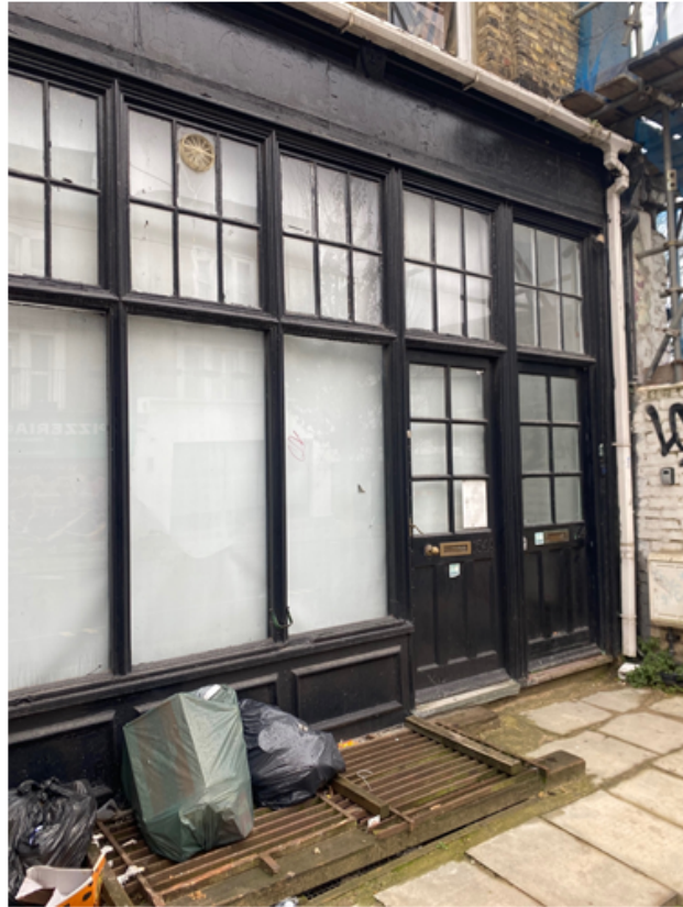
A condition will be attached to secure details of the proposed lightwell cover
