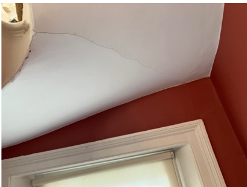
Movement cracks on the staircase
