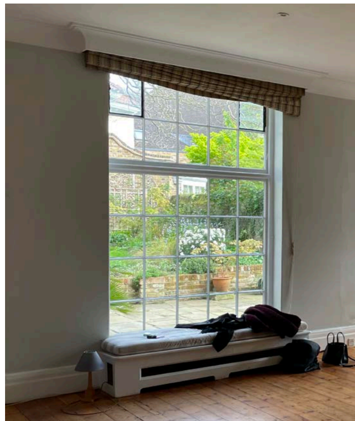
Existing Living Room window in need of repair.
