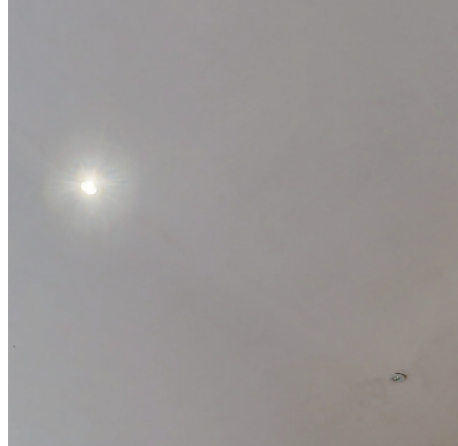
Existing Condition: No Ceiling Rose
