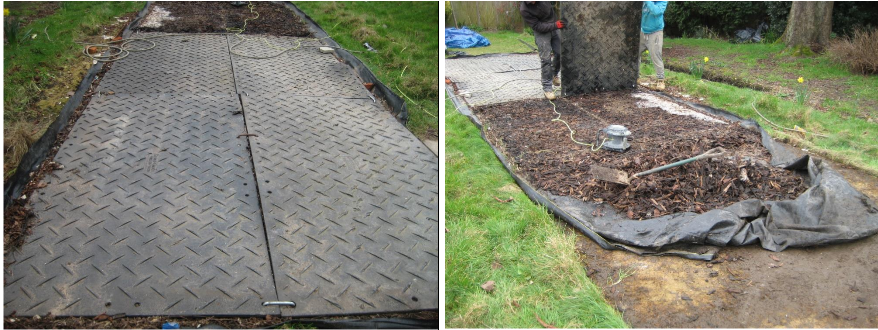
Fig 10 – Temporary ground protection is an effective way of allowing access through the RPA of retained trees. It must be installed prior to any on site activity and maintained for the duration of all works to be effective. Above left Tamla Trees project ground protection in place and above right being removed following the completion of site works. (Note: depending on the length of time it is in place it will adversely affect underlying grass ground cover which will need reseeded/ turfed accordingly)
