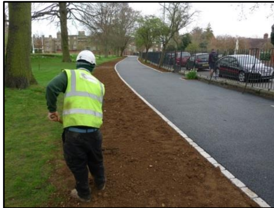
Fig 16 – In the event of 'making good' topsoil will be BS3882 compliant and raked out by hand to no greater depth than 100mm.
