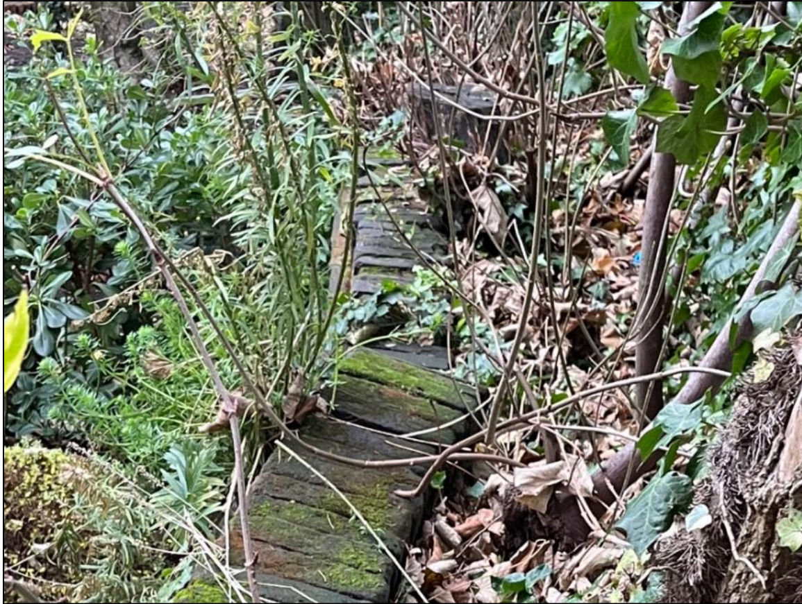
Photograph 3: Buckling of retaining wall evident
