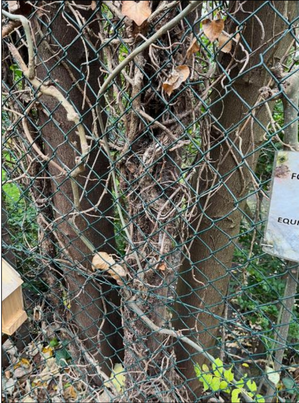
Photograph 4: Typical stem size of trees growing adjacent to wall
