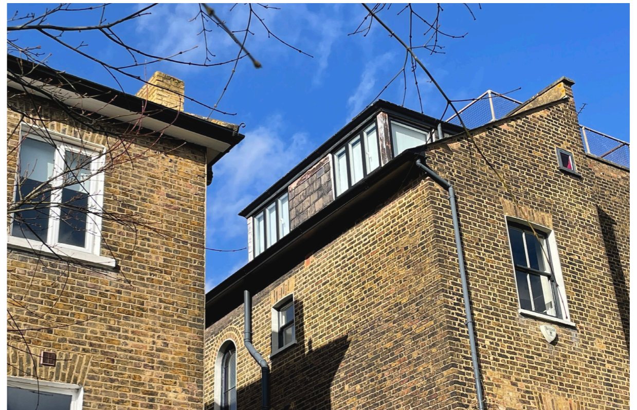
Detail of Neighbouring Dormer Window at 104 Chetwynd Road
