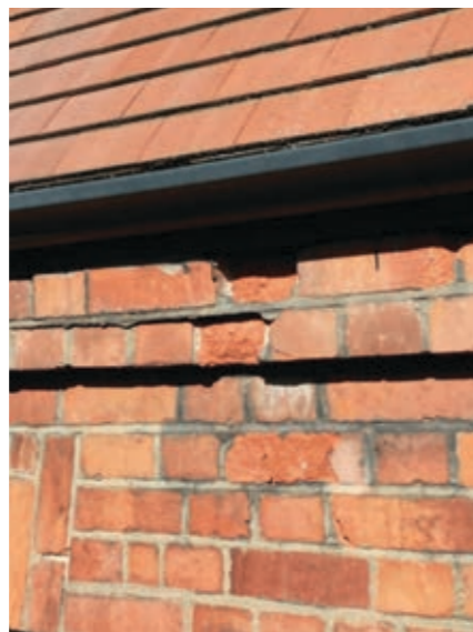
Detail of spalling masonry.
