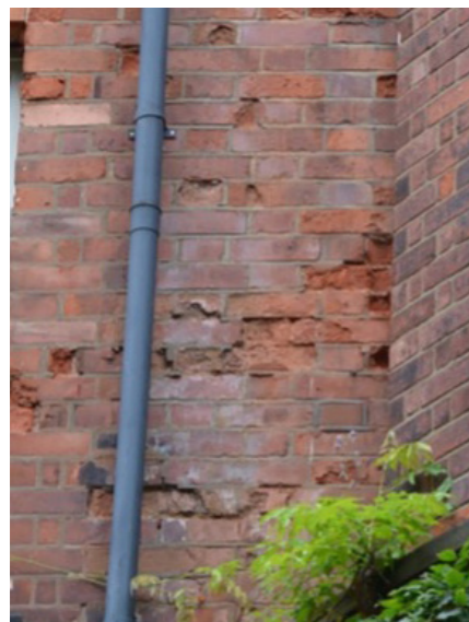
Close up photo of damaged bricks that will need repairing.
