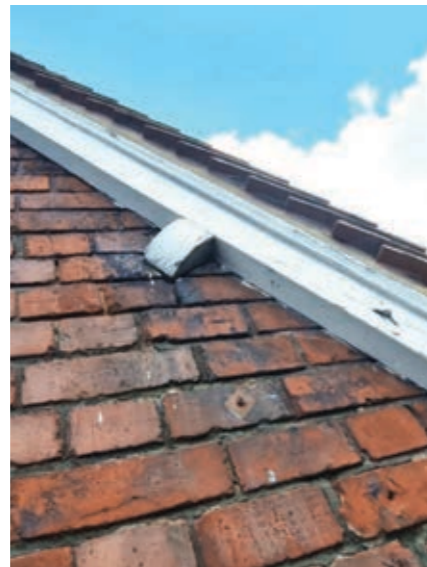
Detail of delimitation of decorative coatings and expansion of timber grain.
