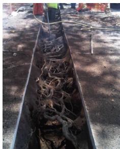
Example imagery of air spade use for implementing utilities beneath root plate (existing)
