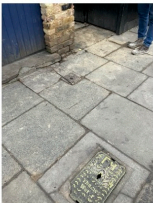
Utilities within highway
