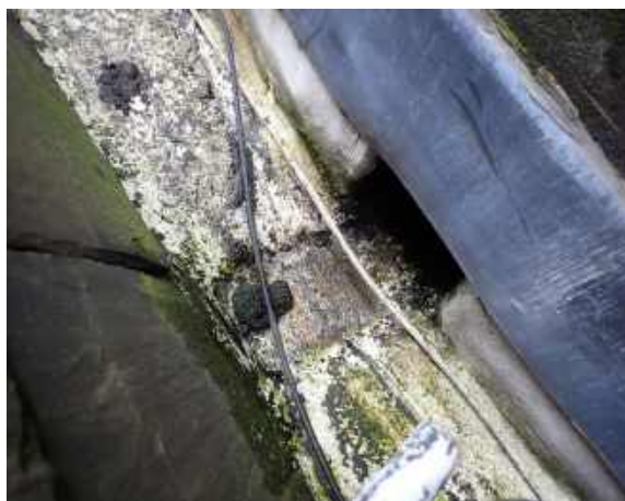
RPT-Figure-23: Rainwater ran away to the south into an apparent internal/embedded downpipe
