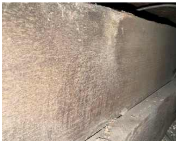
RPT-Figure-29: Saw marks were visible to accessible timber elements at time of survey
