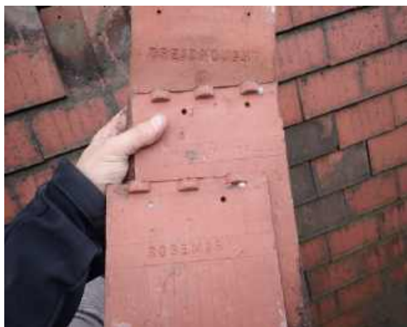
RPT-Figure-15: Several makers stamps/tile types were noted to be used over roof structure
