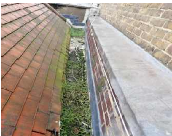
RPT-Figure-39: Rainwater drainage channels were blocked by debris in several areas
