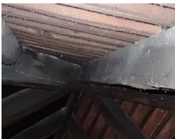
RPT-Figure-35: Interstitial condensation was noted to several timber elements comprising the roof structures in both voids
