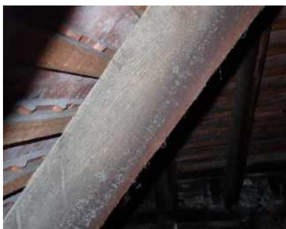
RPT-Figure-36: Interstitial condensation was noted to several timber elements comprising the roof structures in both voids
