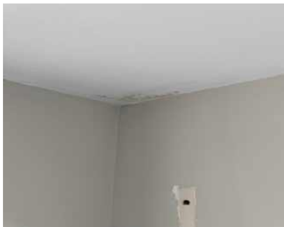
RPT-Figure-44: Damp affected ceiling finishes were noted beneath both roof voids
