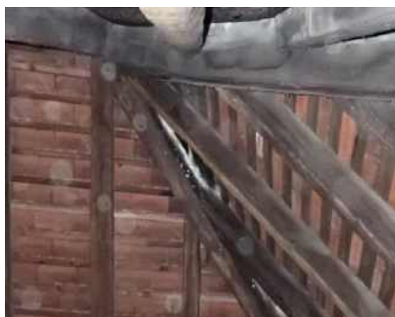
RPT-Figure-46: Wet rot was affecting timber elements in localised instances
