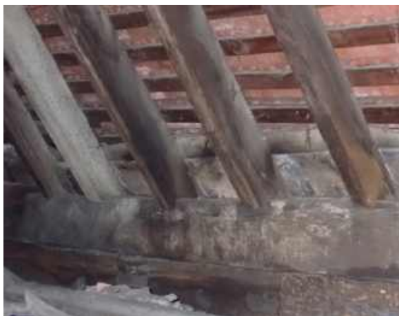
RPT-Figure-26: Birds mouth jointing noted to majority of rafter feet
