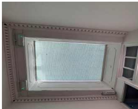
RPT-Figure-19: Limited access to lantern over stairwell at time of survey
