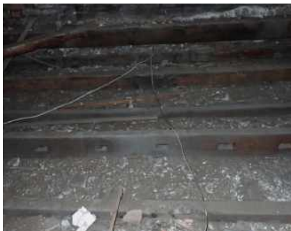
RPT-Figure-38: Debris was noted to the topside of ceiling finishes in both voids
