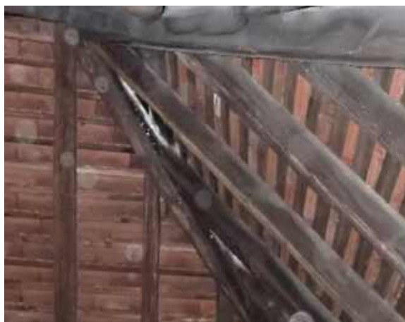
RPT-Figure-34: Wet rot was noted at high level to the east due to external defect
