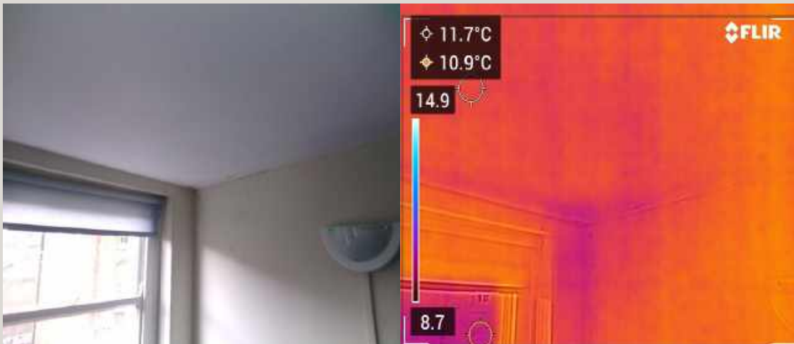
FIG: 58 / Showing both real-light and thermographic image taken from the south-west top-floor for comparative/contextual purposes. Note colder surface temperature was detected towards to high level masonry/interior finishes, indicative of damp conditions
