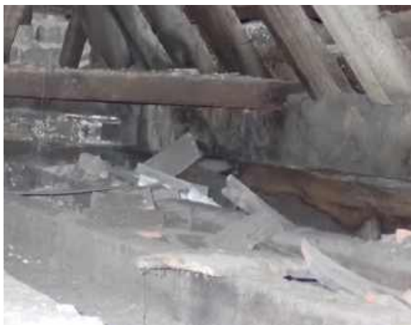
RPT-Figure-37: Debris was noted to the topside of ceiling finishes in both voids
