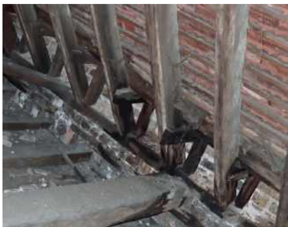
RPT-Figure-33: Clear damp staining was visible to timber elements to the east
