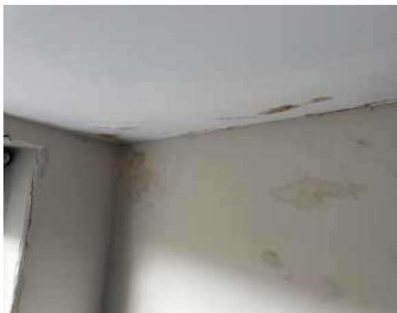
RPT-Figure-43: Damp affected ceiling finishes were noted beneath both roof voids
