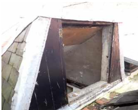
RPT-Figure-42: Roof access hatch doors had completely detached by the time of survey
