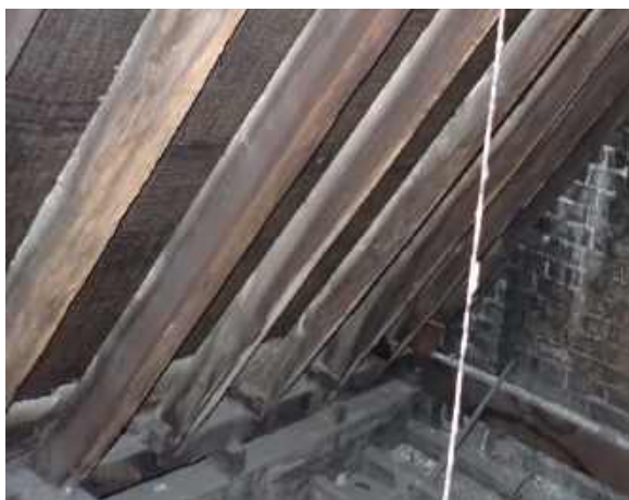
RPT-Figure-14: Non-historic, bituminous underlay was present to west pitch of eastern roof void
