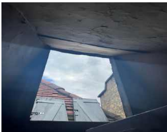
RPT-Figure-41: Failure of the roof access hatch doors left interiors vulnerable to water penetration
