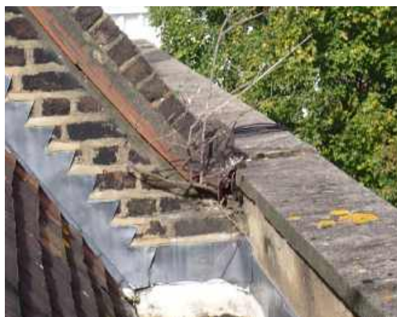
RPT-Figure-40: Rooted plant growth was noted within masonry and through gutter linings
