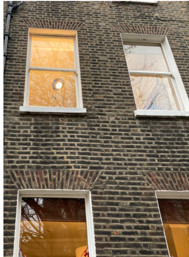
Fig 18. The front façade of No.22 in 2020 showing minor cosmetic refurbishment to the brickwork.
