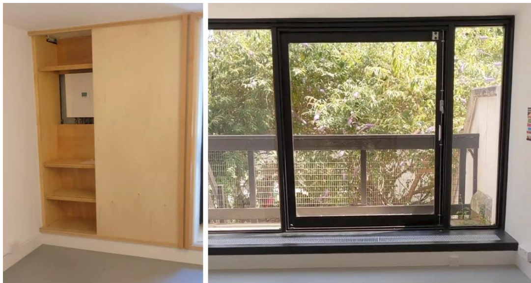
Figure 5 (above): New HIU (left) and refurbished windows (right) in a pilot flat
