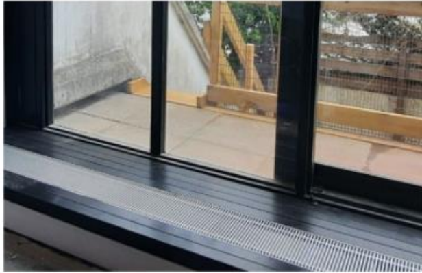
Plinth in living room of 46A pilot flat (B3 Flat Type) with integrated trench heater
