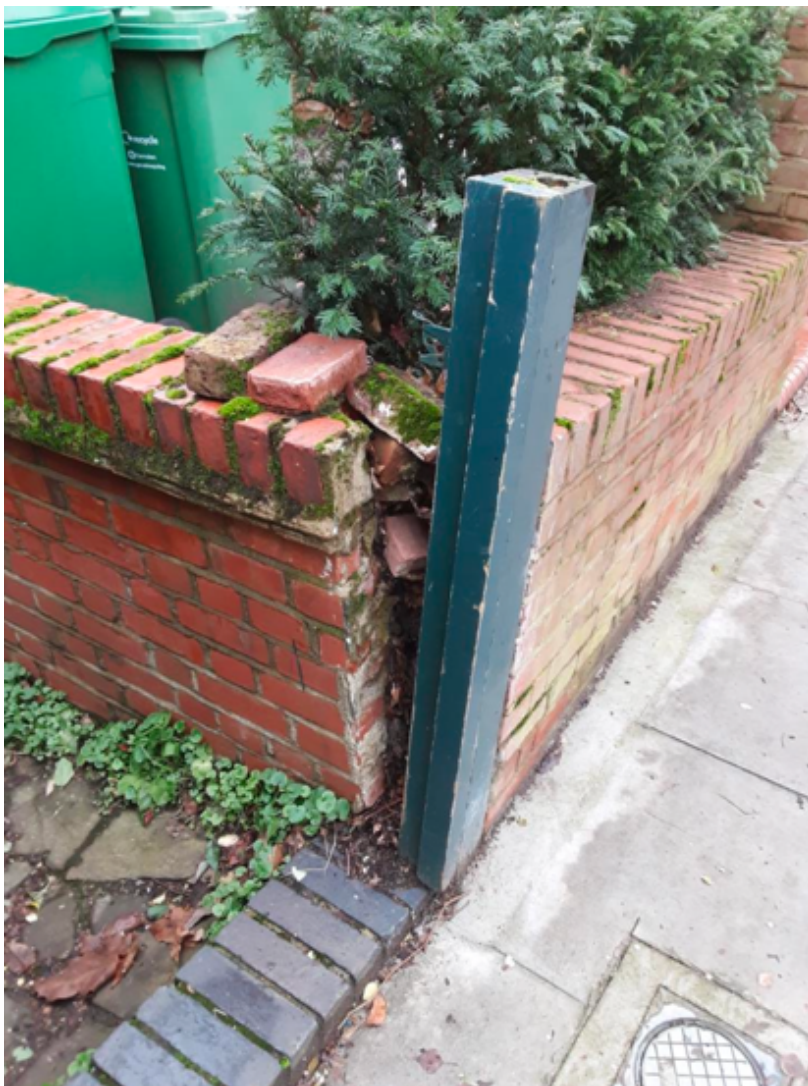
Leaning Boundary / Collapsed Wall (31 / 33 Ferncroft Avenue)
