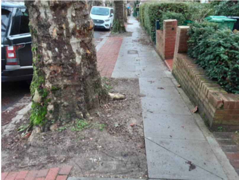
Leaning Boundary / Cracked Wall (31 Ferncroft Avenue / Public Footpath)
