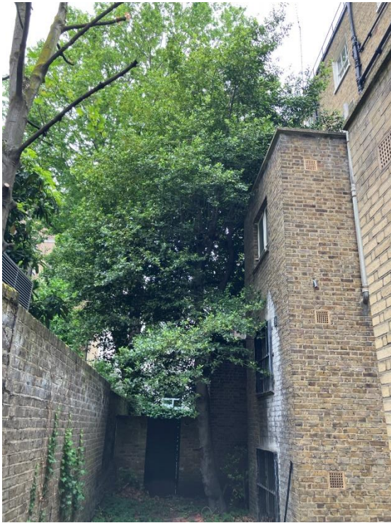
Figure 1: The canopy of T5 growing into the rear of the building.
