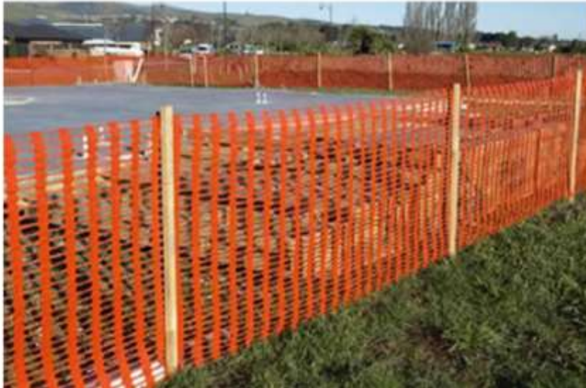
Figure 2: example of high-visibility barrier tape fencing secured with timber stakes (as per AIA report issued)
