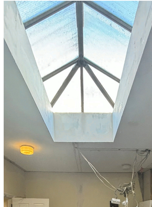
1. Ground Floor. View from below of the existing lantern rooflight, showing visible water marks indicating moisture ingress.
