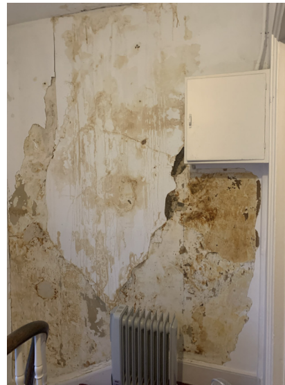
Internal damage from roof leaks
