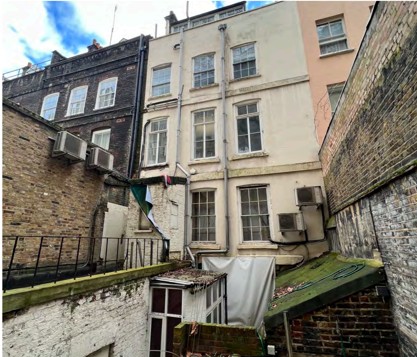
The photograph above illustrates the rear elevation and the associated smaller extensions that have been added over time.
