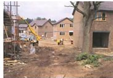
Ground protection is essential to maintain the health of tree roots on construction sites.
