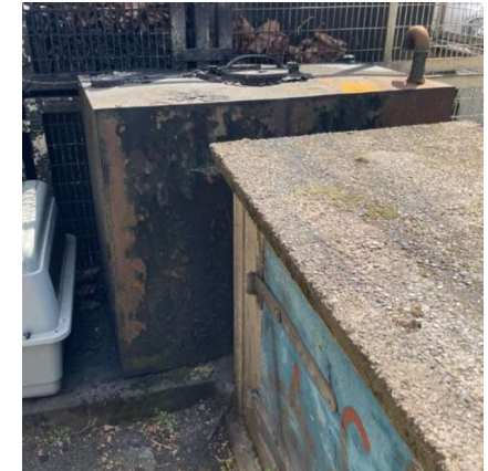
Left: Above ground storage tank with visible staining in roughly the centre west of site
