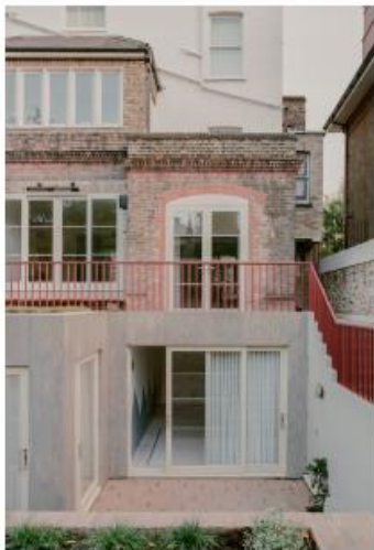
Ground and 1st floors (flat 1), and view of 2nd floor (flat 2) at the rear.
