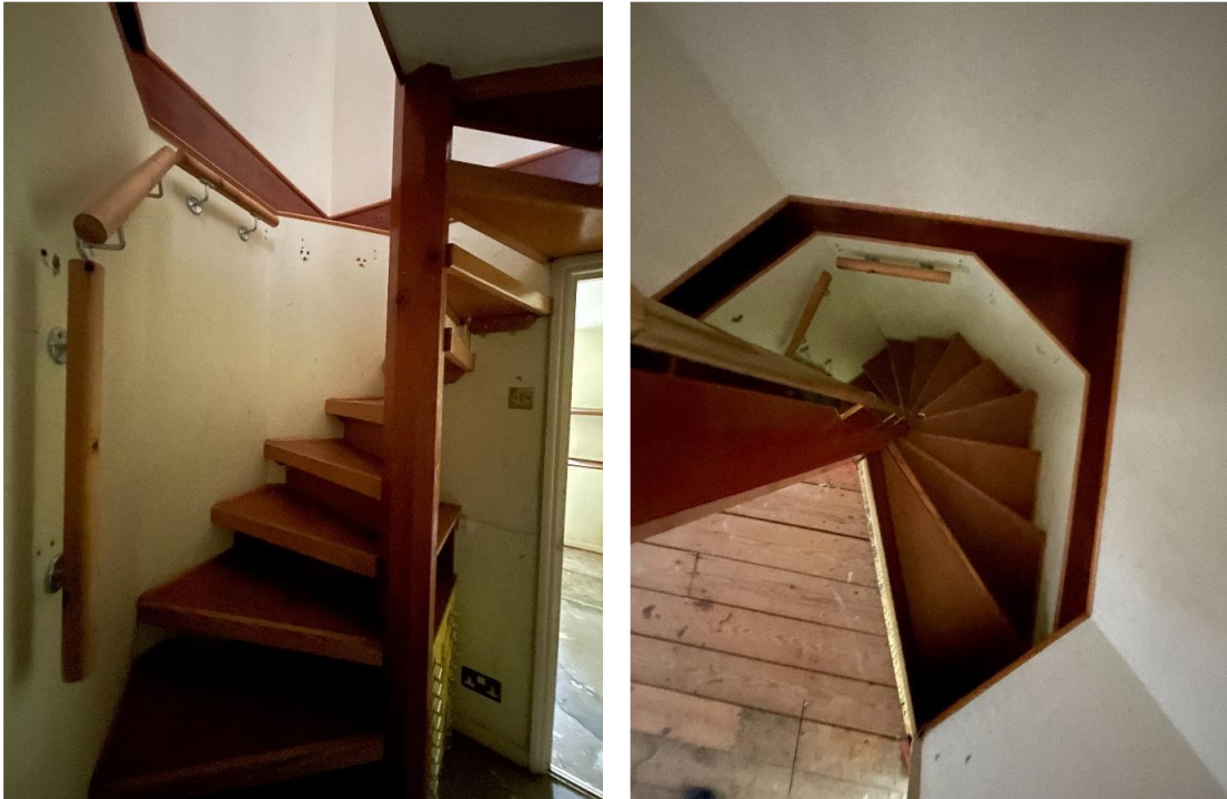
Figure 2 – Substandard spiral staircase
