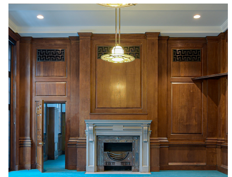
Photographs and elevation example of new grilles sensitively integrated within existing timber panelling in 1.30 Member's Room (below) Drawing not to scale
