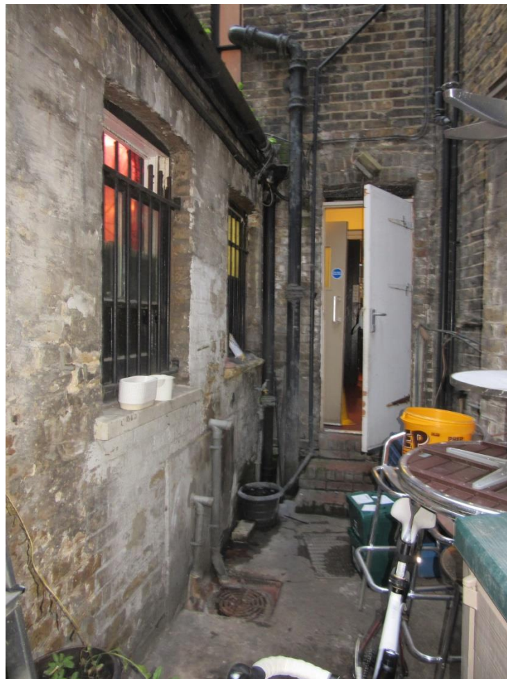
Figure 26: The rear service yard, depicting modern concrete surface, much-altered elevation to the 19 th century outbuilding (rebuilt early 20 th century), and modern door into the pub.
