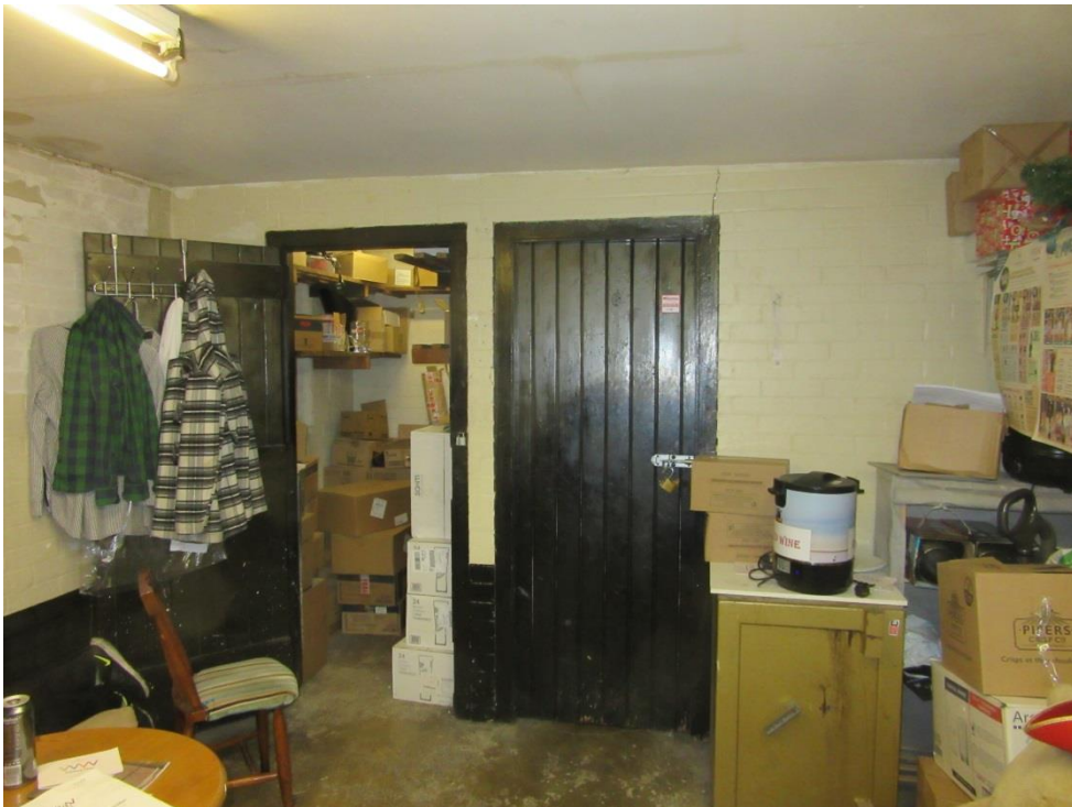
Figure 29: The possibly mid-20 th century basement extension beneath the 1925 extension on Warner Street depicting additional cellarage and barrel chute and later brickwork.
