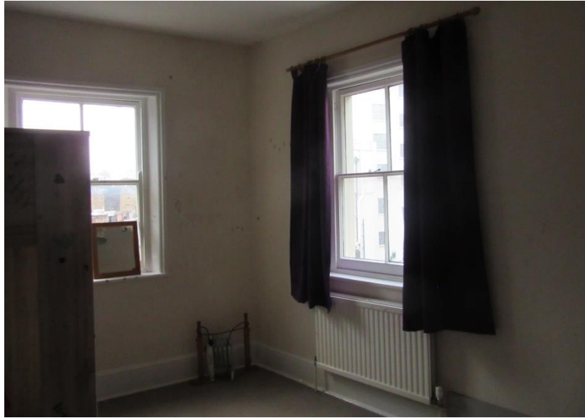
Figure 38: The dimensions of the second floor rooms appear to be original and are typically plain with no cornicing or elaborate joinery; the fireplaces have been removed and boarded over.
