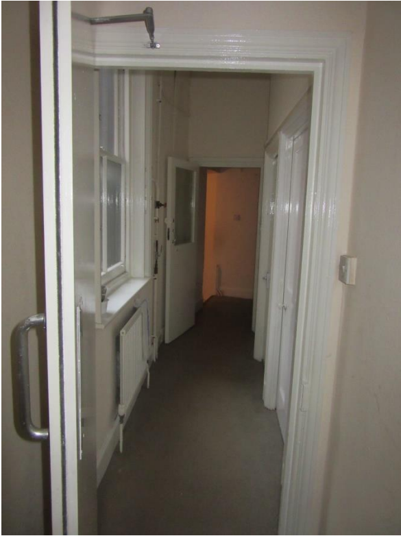
Figure 35: The first floor corridor to the rooms within the 1925 extension taken from the east room.
