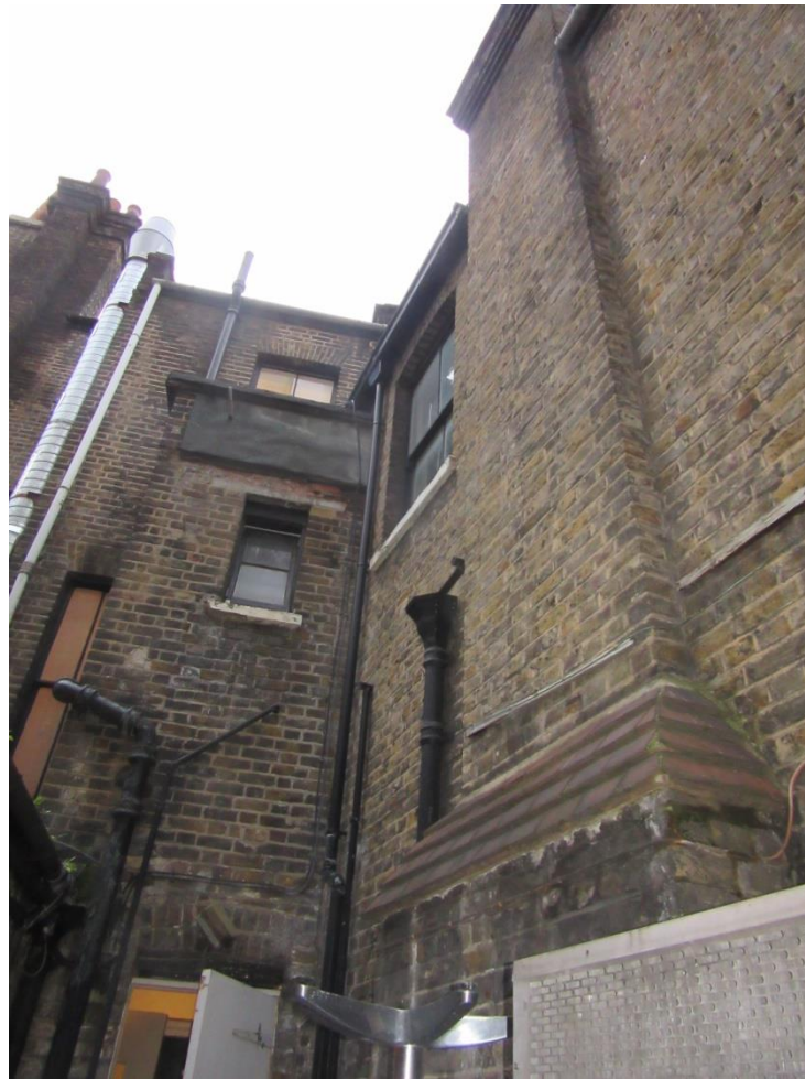
Figure 27: The rear east and south elevations of the 1870s building and 1925 extension, illustrating the unsightly accretion of services, poor-quality alterations to the “stair tower” and dominance of the 1920s chimney stack.
