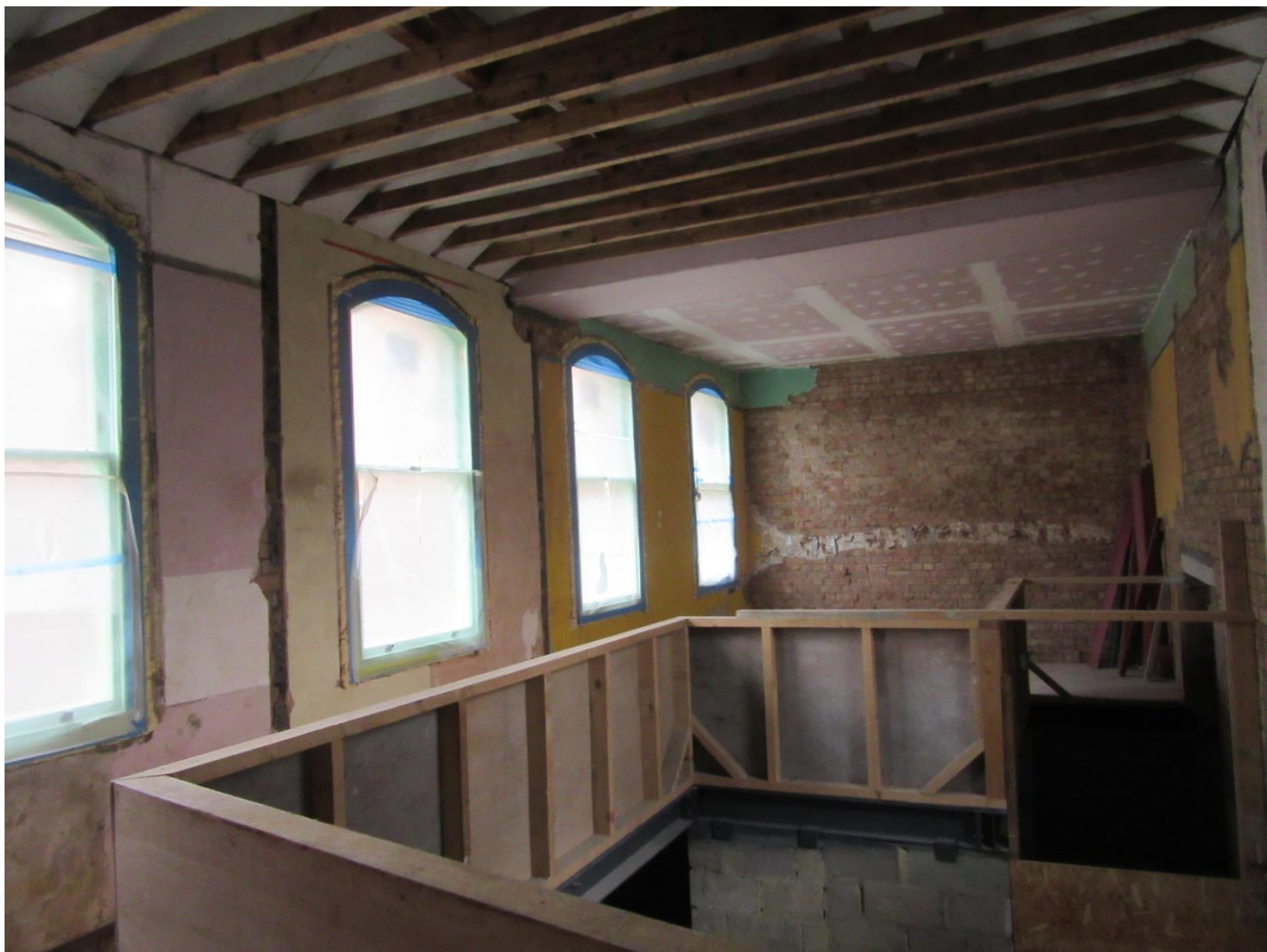
Figure 6: The first floor of the Warner Street extension, illustrating the unfinished space and incomplete consented staircase with doorway into the new 2-storey rear “toilet” extension.
