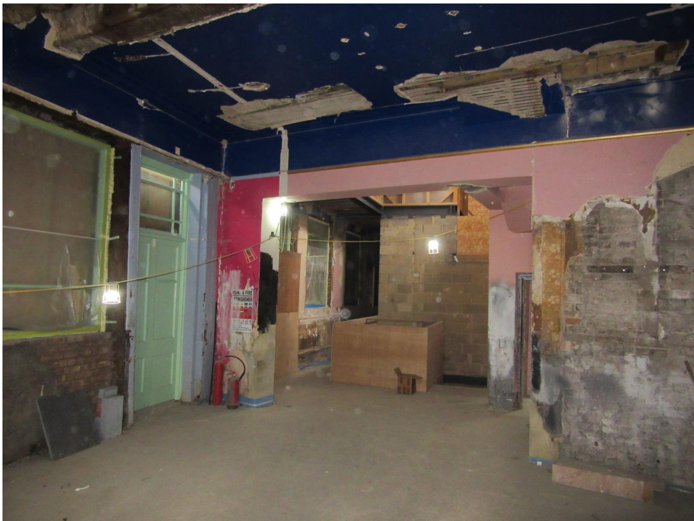
Figure 2: The former bar area looking into the Warner Street extension with consented removed 1930s staircase and bar, and new partially completed staircase and modern concrete floor.
