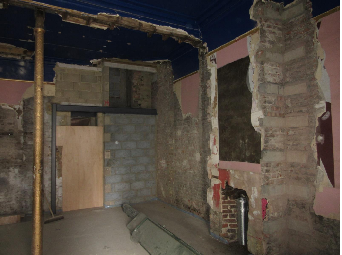
Figure 4: The rear of the former bar area, with blockwork filling the space formerly occupied by the dumb waiter.
