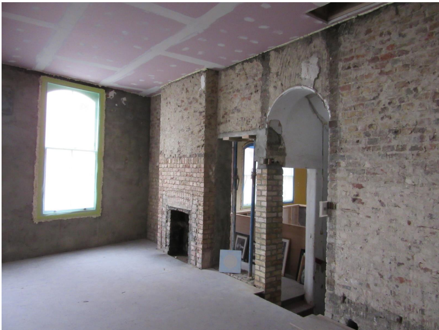
Figure 7: The rear part of the first floor of the 1870s building with removed partitions, consented new doorway adjacent to the chimneybreast and incomplete finishes.
