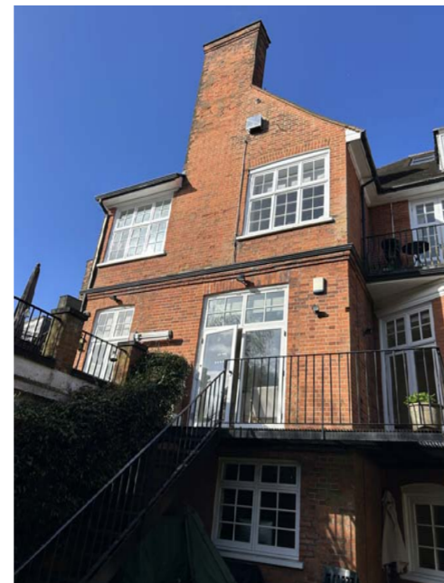
The existing black steel steps and balcony which wraps around the rear outrigger
