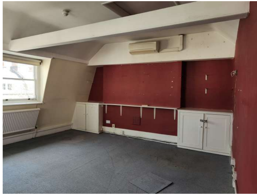
Figure 27: Third floor NB ceiling raised and tie beam of truss boxed in.
