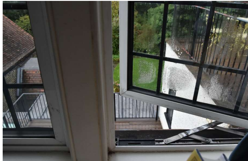
Detail of blown seals to double glazed units.
