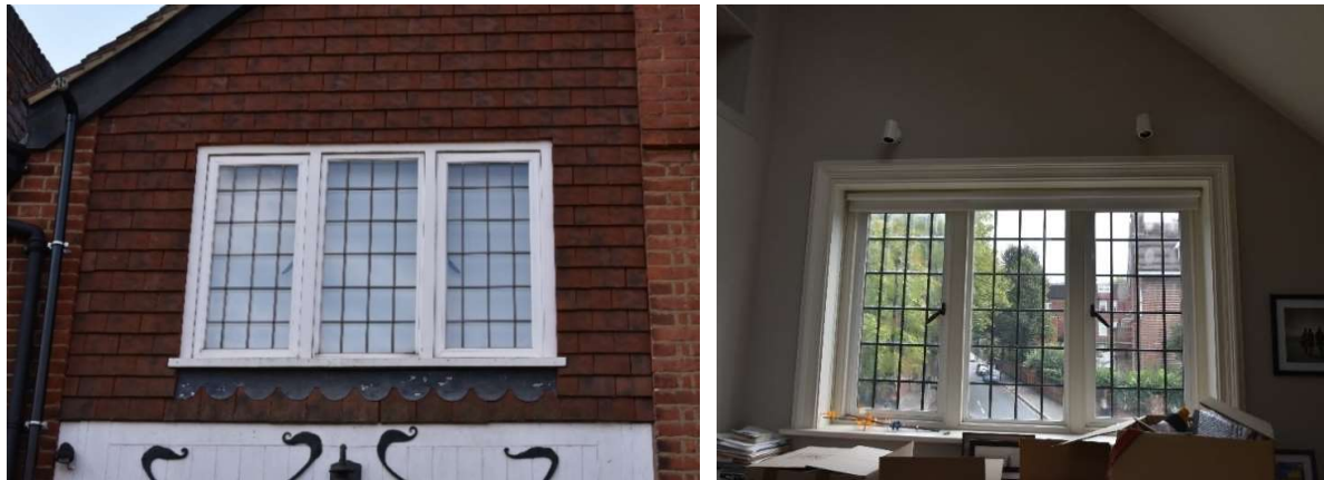
Double glazed windows to new study where sealed units have blown exterior and internal views.
