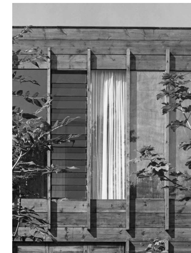
Aim to restore roof junction detail to original, as pictured above in photo by Arnold Behr (1961)
